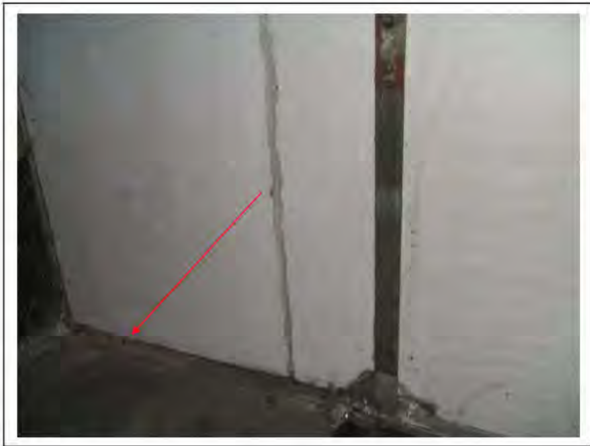
FIGURE 195: PRESUMED ASBESTOS IN RESIDUE BELOW SUPALUX ON BEAM IN VENT SHAFT , 3/902 - DESCRIPTION & RESULT OF ASSESSMENT (SAMPLE REF. P1&2(60))
