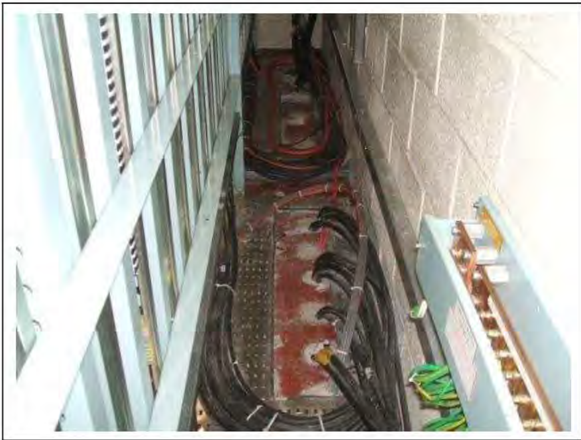
FIGURE 134: PRESUMED ASBESTOS IN POSSIBLE CAULKING IN SER, 3/371 - DESCRIPTION & RESULT OF ASSESSMENT (SAMPLE REF. P1&2(55))
