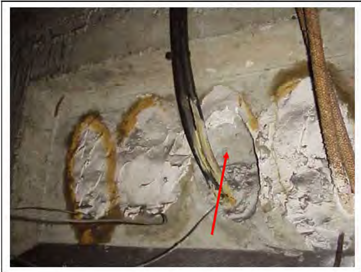
FIGURE 122: CONFIRMED ASBESTOS IN CABLE SLEEVES IN VICTORIA LINE, PLATFORM 2 INVERT, 3/262, DOWN HATCH NEAR 3/712 - DESCRIPTION & RESULT OF ASSESSMENT (SAMPLE REF. 034219/3)
