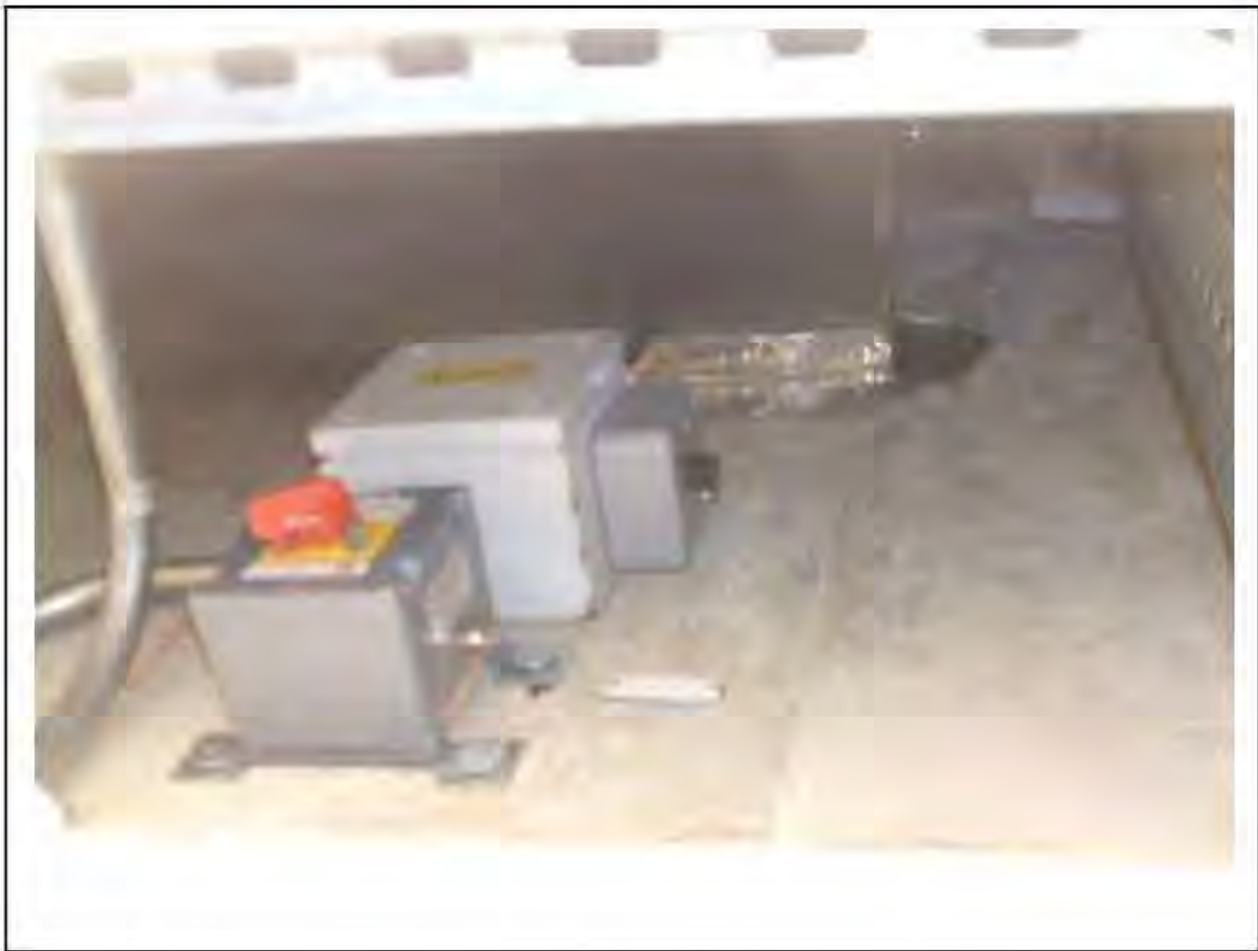
FIGURE 70: PRESUMED ASBESTOS IN RESIDUES IN VENT ACCESS , 2/953 - DESCRIPTION & RESULT OF ASSESSMENT (SAMPLE REF. P1&2(53))
