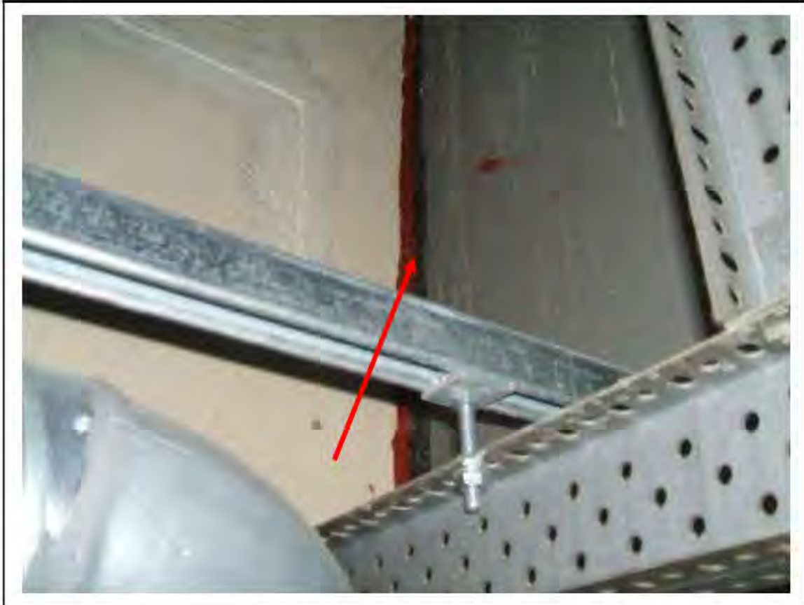
FIGURE 8: PRESUMED ASBESTOS IN SUPALUX BOXING CLADDING POSSIBLE RESIDUES IN WALL AROUND BEAM IN MESS ROOM , 2/032 - DESCRIPTION & RESULT OF ASSESSMENT (SAMPLE REF. P1&2(8))
