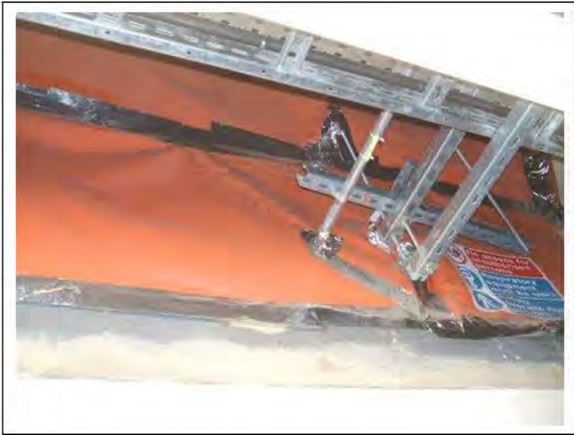
FIGURE 42: PRESUMED ASBESTOS IN VOID OVER ROOM 2/LFI AND ESCALATORS IN PASSAGE , 2/238 - DESCRIPTION & RESULT OF ASSESSMENT (SAMPLE REF. P1&2(29))
