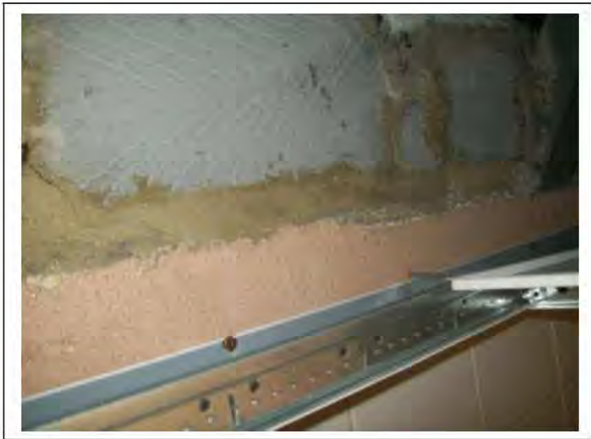
FIGURE 103: KNOWN ASBESTOS IN CELLACTITE CORRUGATED SHEETING IN CORRIDOR, 3/237 - DESCRIPTION & RESULT OF ASSESSMENT (SAMPLE REF. K1(24))
