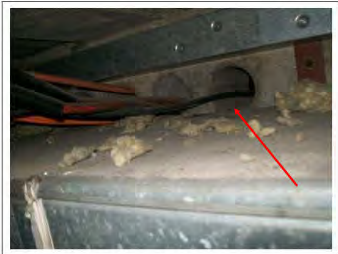
FIGURE 185: CONFIRMED ASBESTOS IN DUCTS TO DIVIDING WALL IN CABLE SHAFT, 3/786 - DESCRIPTION & RESULT OF ASSESSMENT (SAMPLE REF. SAME AS 120445/190812/01)
