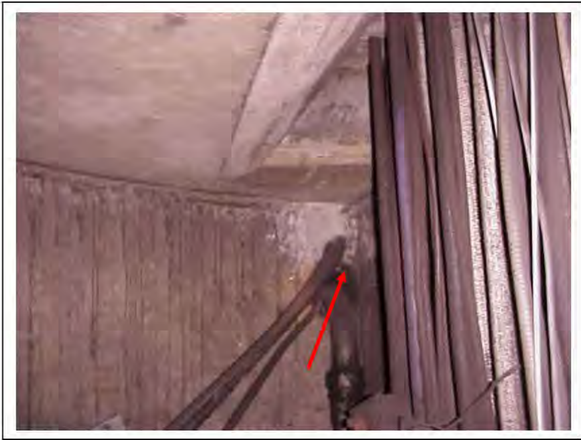
FIGURE 130: CONFIRMED ASBESTOS IN CABLE SLEEVES IN VICTORIA LINE, PLATFORM 2 INVERT, 3/262, OTHER END 3/706 - DESCRIPTION & RESULT OF ASSESSMENT (SAMPLE REF. SAME AS 034219/5)
