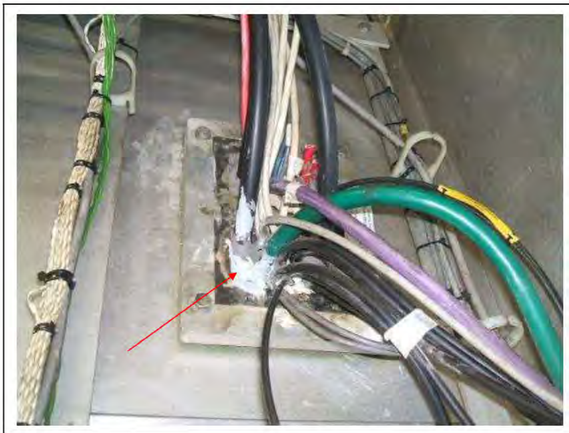
FIGURE 169: KNOWN ASBESTOS IN BRAIDED CABLE STUB IN RELAY ROOM , 3/712 - DESCRIPTION & RESULT OF ASSESSMENT (SAMPLE REF. K1(44))
