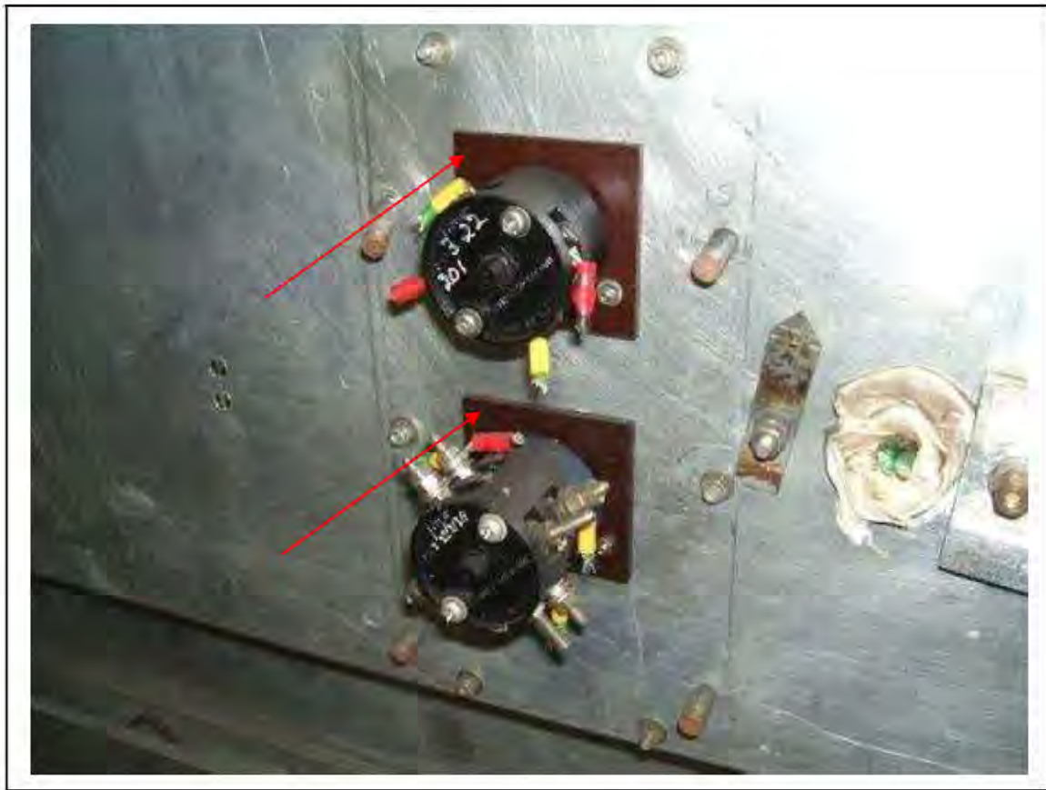
FIGURE 167: STRONGLY PRESUMED ASBESTOS IN SILUMINITE IN RELAY ROOM , 3/711 - DESCRIPTION & RESULT OF ASSESSMENT (SAMPLE REF. SP1(18))
