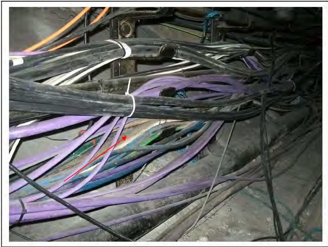
FIGURE 188: KNOWN ASBESTOS IN BRAIDED CABLES IN CABLE SHAFT , 3/787 - DESCRIPTION & RESULT OF ASSESSMENT (SAMPLE REF. K1(48))
