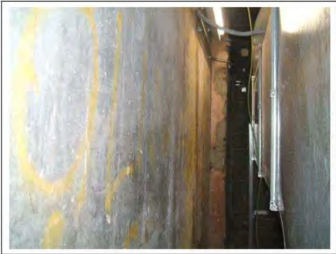
FIGURE 64: PRESUMED ASBESTOS IN RESIDUES BEHIND REAR FALSE WALL IN SERVICE VOID , 2/902 - DESCRIPTION & RESULT OF ASSESSMENT (SAMPLE REF. P1&2(48))
