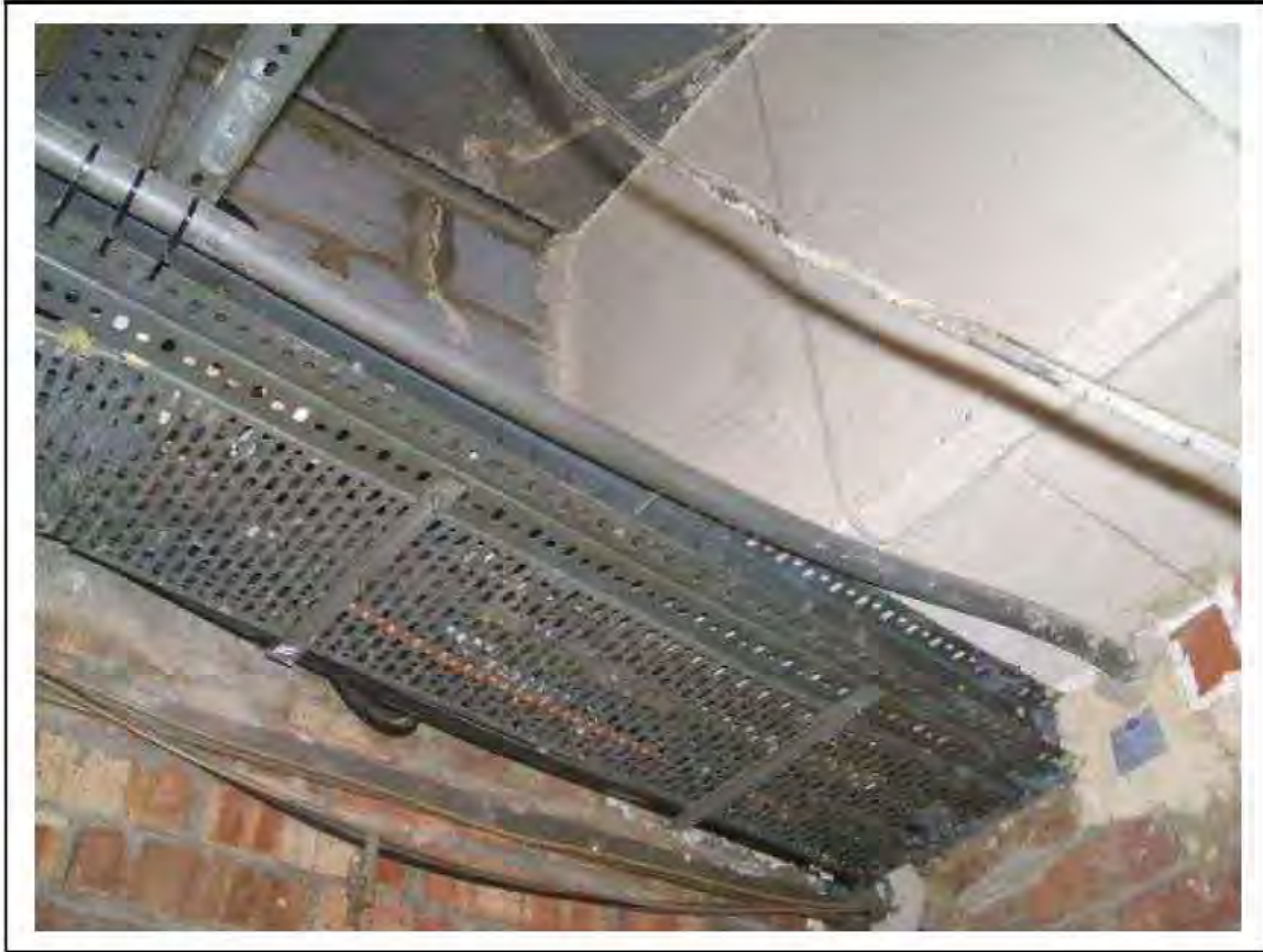
FIGURE 50: PRESUMED ASBESTOS IN RESIDUE IN WALL BETWEEN 2/407 AND ESCALATOR INCLINE 2/171 IN STORE, 2/407 - DESCRIPTION & RESULT OF ASSESSMENT (SAMPLE REF. P1&2(36))
