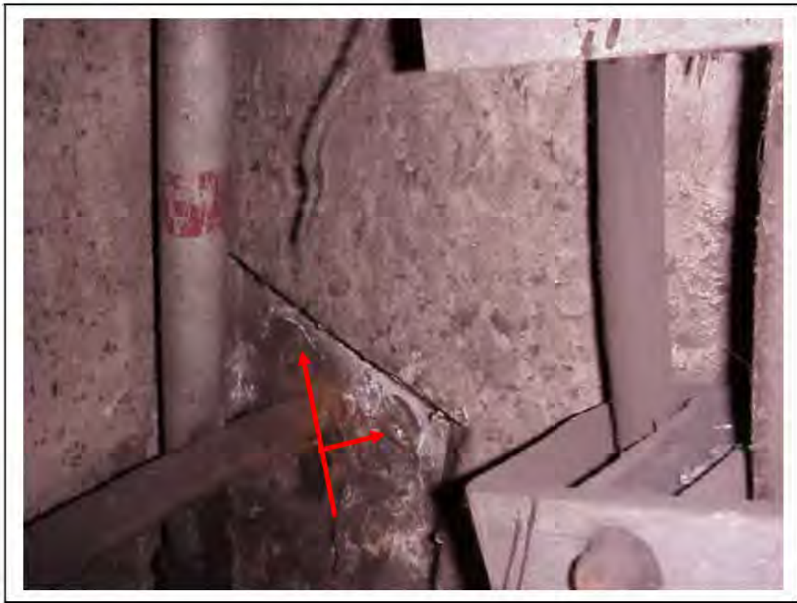
FIGURE 131: CONFIRMED ASBESTOS IN CABLE SLEEVES IN VICTORIA LINE, PLATFORM 2 INVERT, 3/262, OTHER END 3/706 - DESCRIPTION & RESULT OF ASSESSMENT (SAMPLE REF. SAME AS 034219/5)
