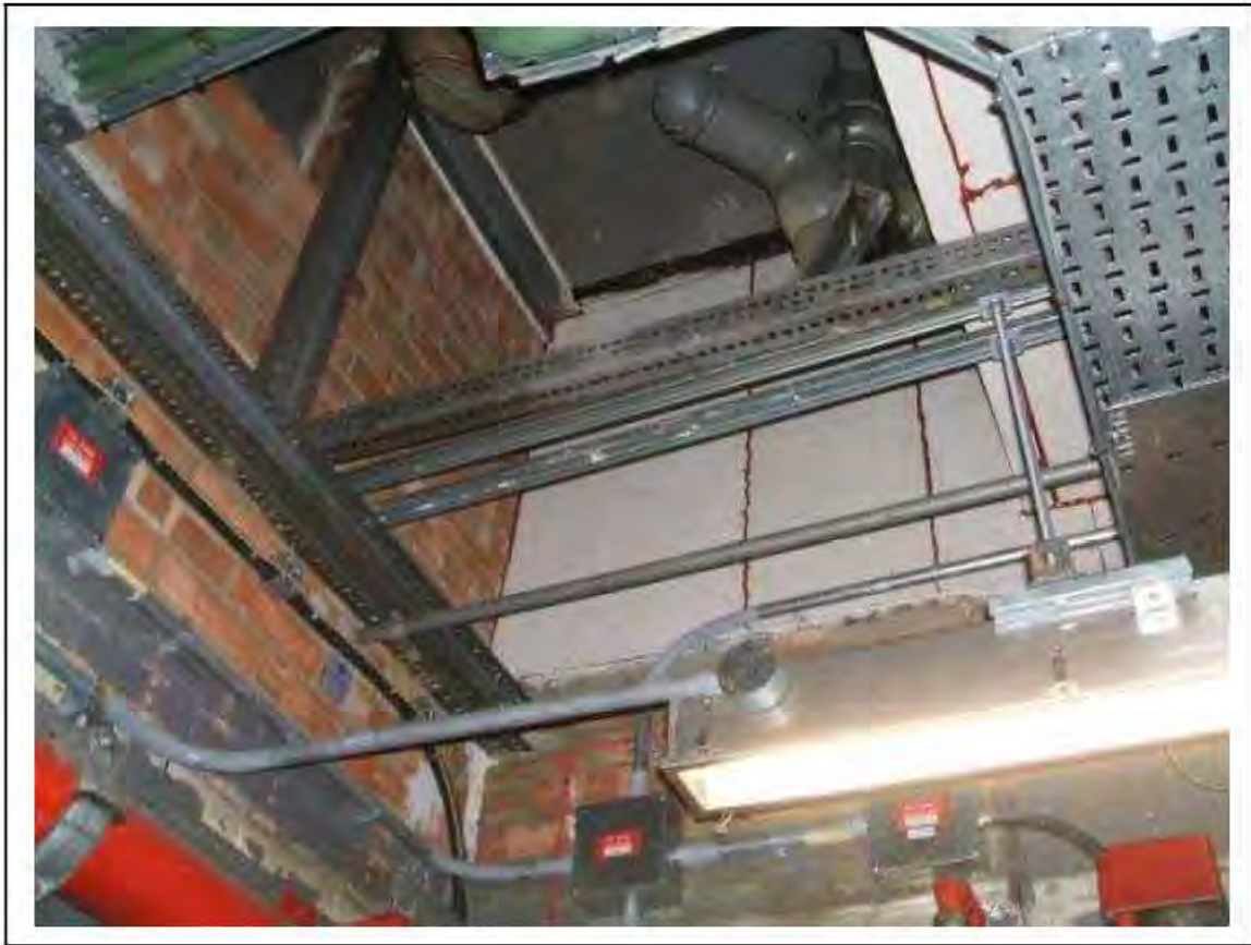
FIGURE 16: PRESUMED ASBESTOS IN RESIDUE WITHIN CAVITY WALL BENEATH BEAM S9 IN UMC ACCESS , 2/151 - DESCRIPTION & RESULT OF ASSESSMENT (SAMPLE REF. P1&2(15))
