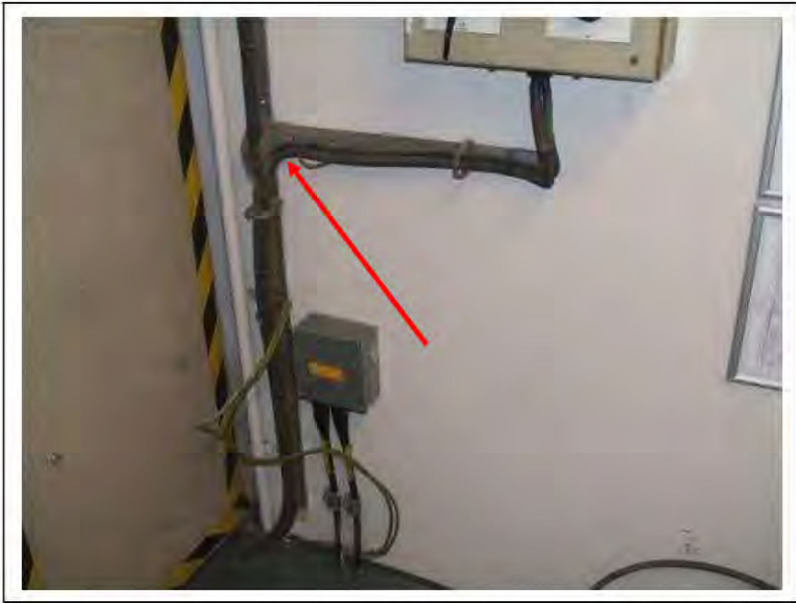
FIGURE 141: KNOWN ASBESTOS IN BRAIDED CABLES IN SWITCH ROOM E5, 3/662 - DESCRIPTION & RESULT OF ASSESSMENT (SAMPLE REF. K1(35))
