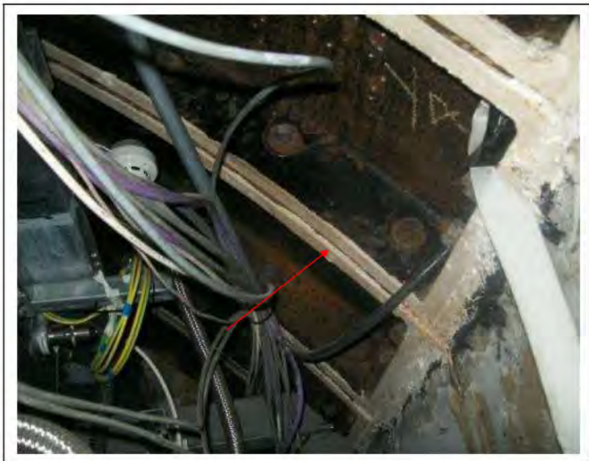
FIGURE 102: CONFIRMED ASBESTOS IN CAULKING IN CORRIDOR, 3/237 - DESCRIPTION & RESULT OF ASSESSMENT (SAMPLE REF. SAME AS 120445/150812/03)
