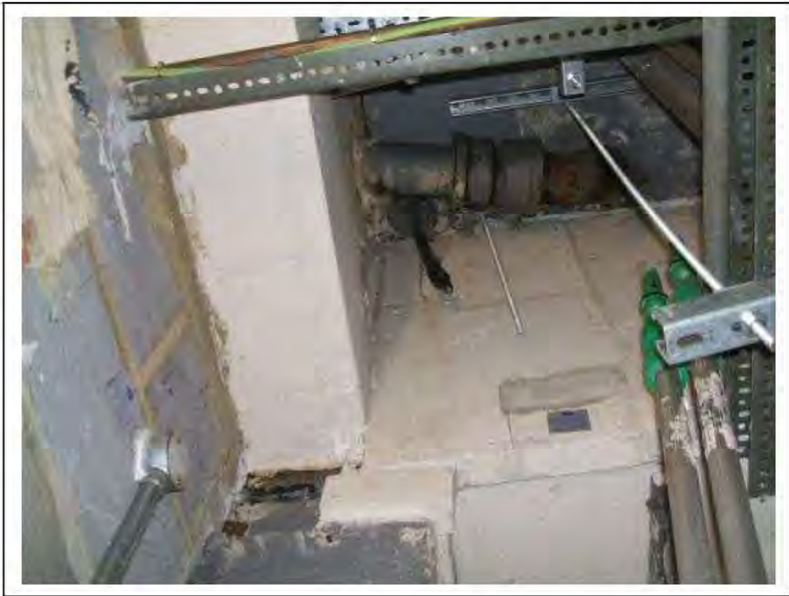
FIGURE 49: PRESUMED ASBESTOS IN RESIDUES WHERE PIPE GOES THROUGH THE CEILING S10 IN STORE, 2/407 - DESCRIPTION & RESULT OF ASSESSMENT (SAMPLE REF. P1&2(35))
