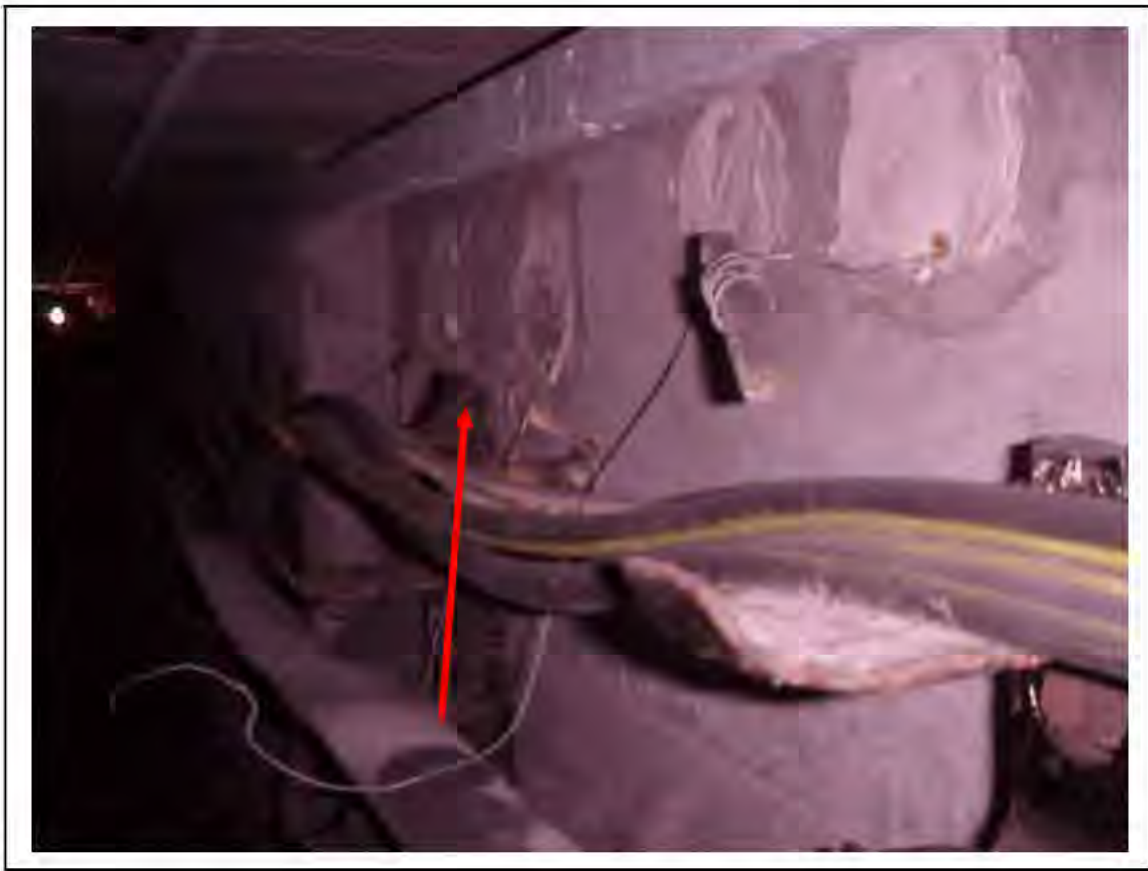
FIGURE 113: KNOWN ASBESTOS IN CABLES IN VICTORIA LINE, PLATFORM 1 INVERT, 3/261, 30M UP - DESCRIPTION & RESULT OF ASSESSMENT (SAMPLE REF. K1(27))
