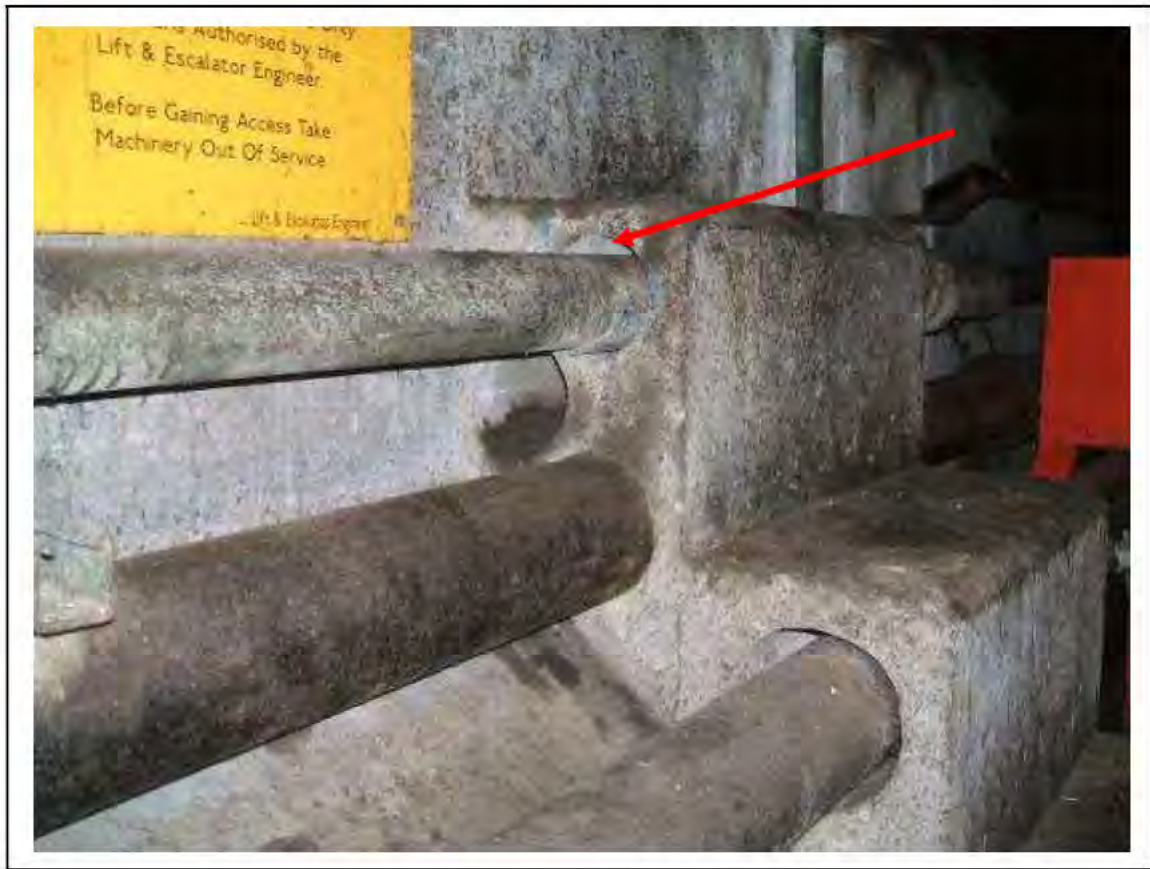
FIGURE 81: CONFIRMED ASBESTOS IN DUCTS IN LMC, 3/161 - DESCRIPTION & RESULT OF ASSESSMENT (SAMPLE REF. SAME AS 120445/130812/1)
