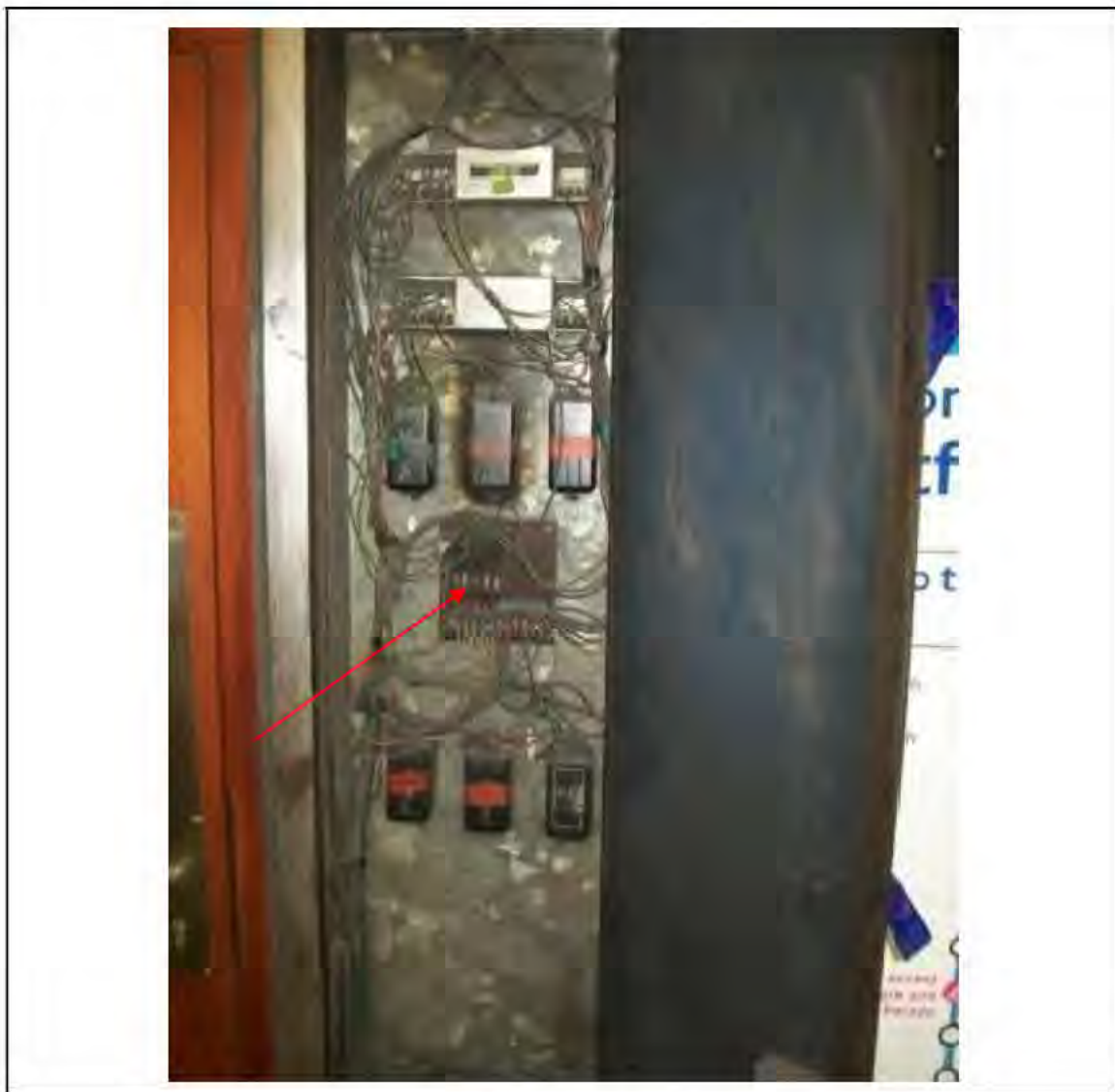
FIGURE 145: STRONGLY PRESUMED ASBESTOS IN SILUMINITE PANEL IN LIGHTING CUPBOARD , 3/669 - DESCRIPTION & RESULT OF ASSESSMENT (SAMPLE REF. SP1(3))
