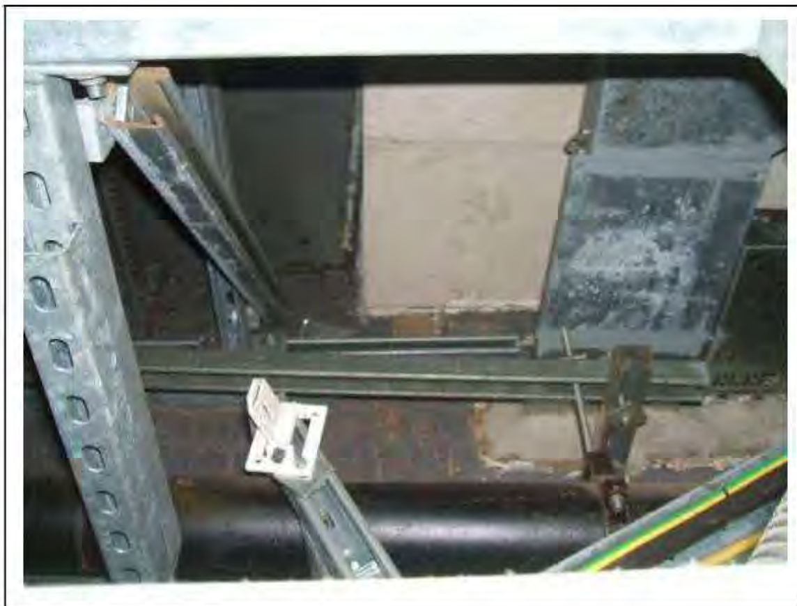
FIGURE 34: PRESUMED ASBESTOS IN RESIDUES BELOW ESCALATOR INCLINE , 2/171 - DESCRIPTION & RESULT OF ASSESSMENT (SAMPLE REF. P1&2(22))
