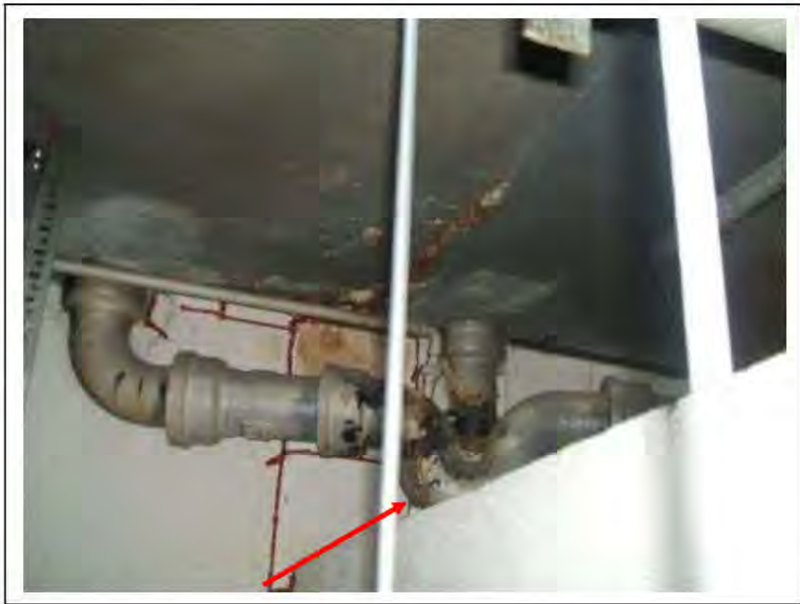
FIGURE 13: PRESUMED ASBESTOS IN RESIDUE AROUND SOIL PIPE IN UMC ACCESS , 2/151 - DESCRIPTION & RESULT OF ASSESSMENT (SAMPLE REF. P1&2(61))
