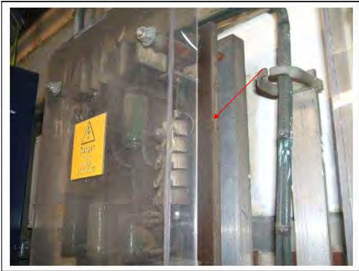
FIGURE 142: STRONGLY PRESUMED ASBESTOS IN SILUMINITE BOARD IN SWITCH ROOM E5, 3/662 - DESCRIPTION & RESULT OF ASSESSMENT (SAMPLE REF. SP1(1))
