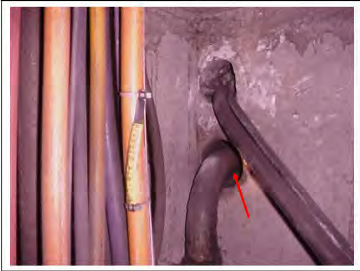
FIGURE 116: CONFIRMED ASBESTOS IN CABLE SLEEVES IN VICTORIA LINE, PLATFORM 1 INVERT, 3/261, OTHER END 3/706 - DESCRIPTION & RESULT OF ASSESSMENT (SAMPLE REF. SAME AS 034219/7,8,10)
