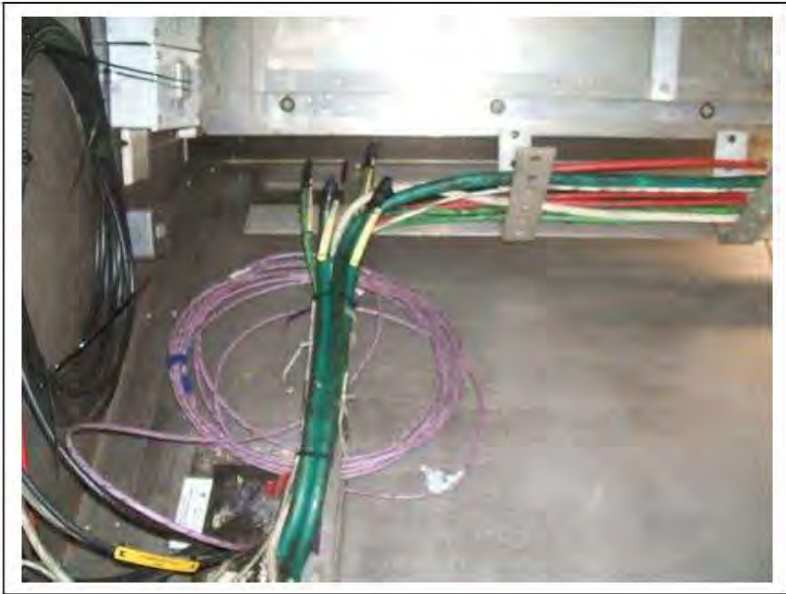
FIGURE 159: KNOWN ASBESTOS IN BRAIDED CABLE IN IMR (CORRIDOR TO PLATFORM 2), 3/706 - DESCRIPTION & RESULT OF ASSESSMENT (SAMPLE REF. K1(41))
