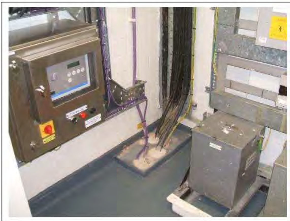
FIGURE 60: PRESUMED ASBESTOS IN CEMENT DUCTS IN SWITCH ROOM E7, 2/667 - DESCRIPTION & RESULT OF ASSESSMENT (SAMPLE REF. P1(7))
