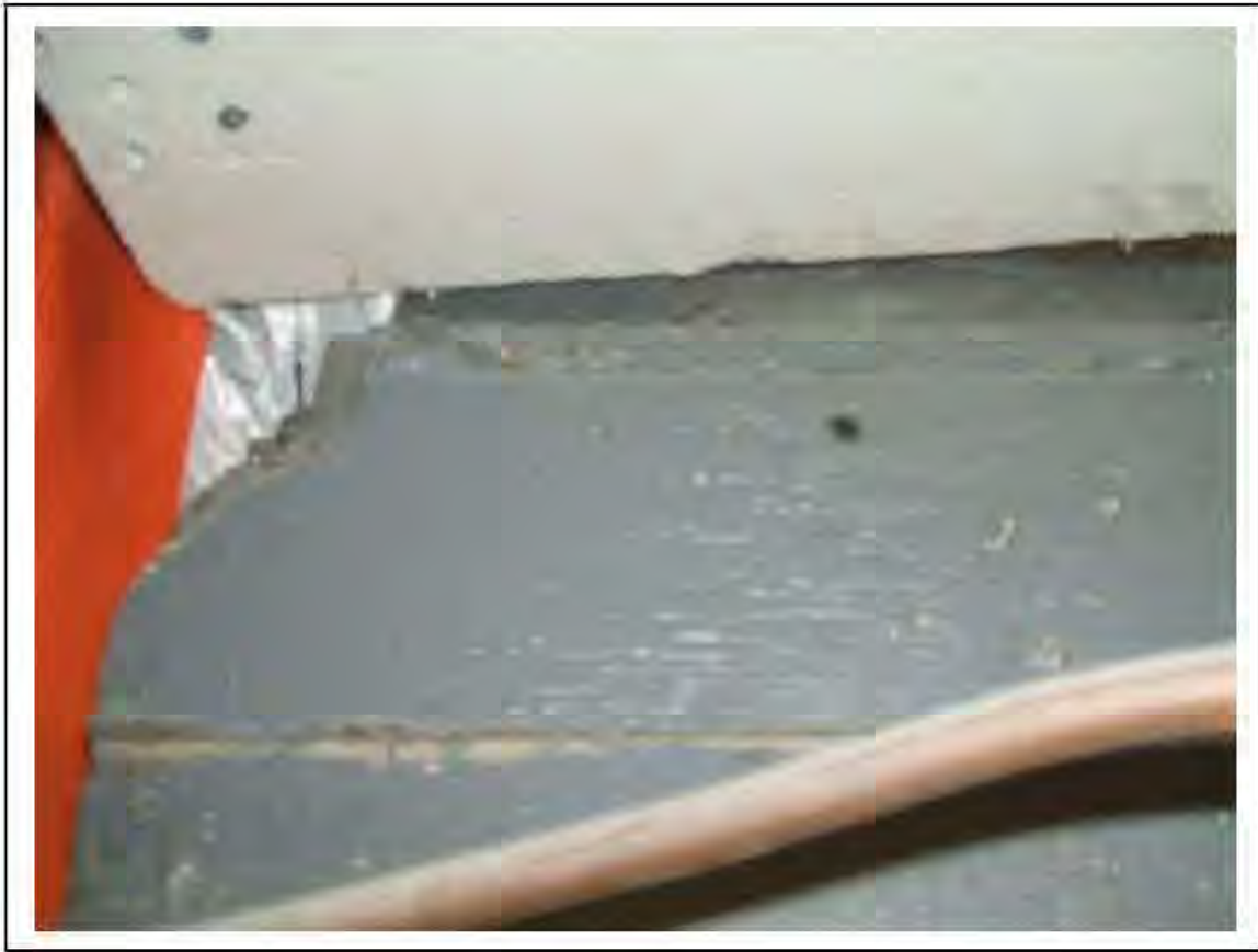
FIGURE 44: PRESUMED ASBESTOS IN BEAM FIBREBOARD CLAD OVER 2/668 AND END OF 2/407 IN PASSAGE , 2/238 - DESCRIPTION & RESULT OF ASSESSMENT (SAMPLE REF. P1&2(31))
