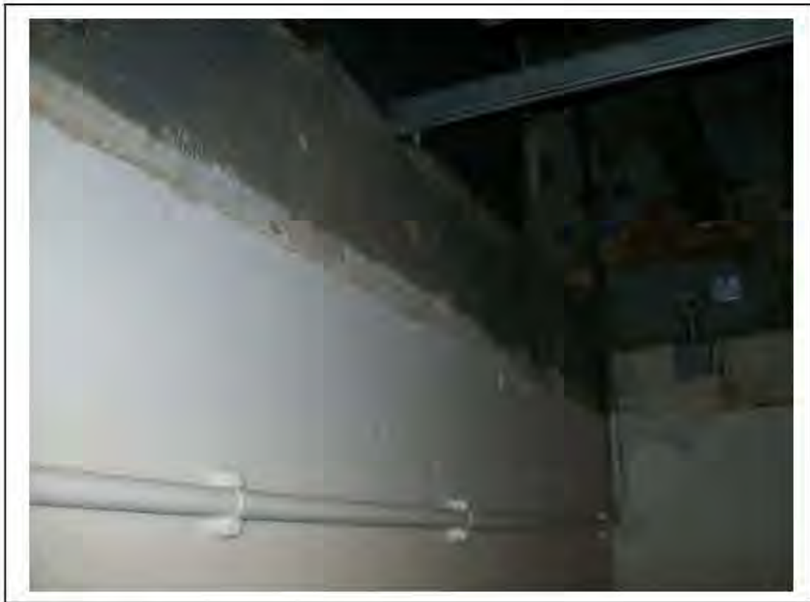
FIGURE 48: PRESUMED ASBESTOS IN RESIDUAL SPRAY INSULATION WITHIN CAVITY IN SVC, 2/401 - DESCRIPTION & RESULT OF ASSESSMENT (SAMPLE REF. P1&2(34))
