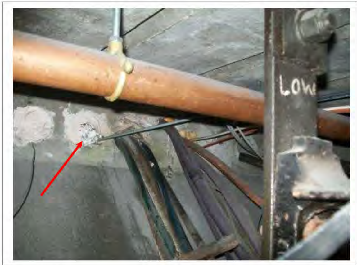
FIGURE 90: CONFIRMED ASBESTOS IN CABLE DUCTS IN PASSAGE FLOOR, 3/205 - DESCRIPTION & RESULT OF ASSESSMENT (SAMPLE REF. SAME AS 120445/190812/01)
