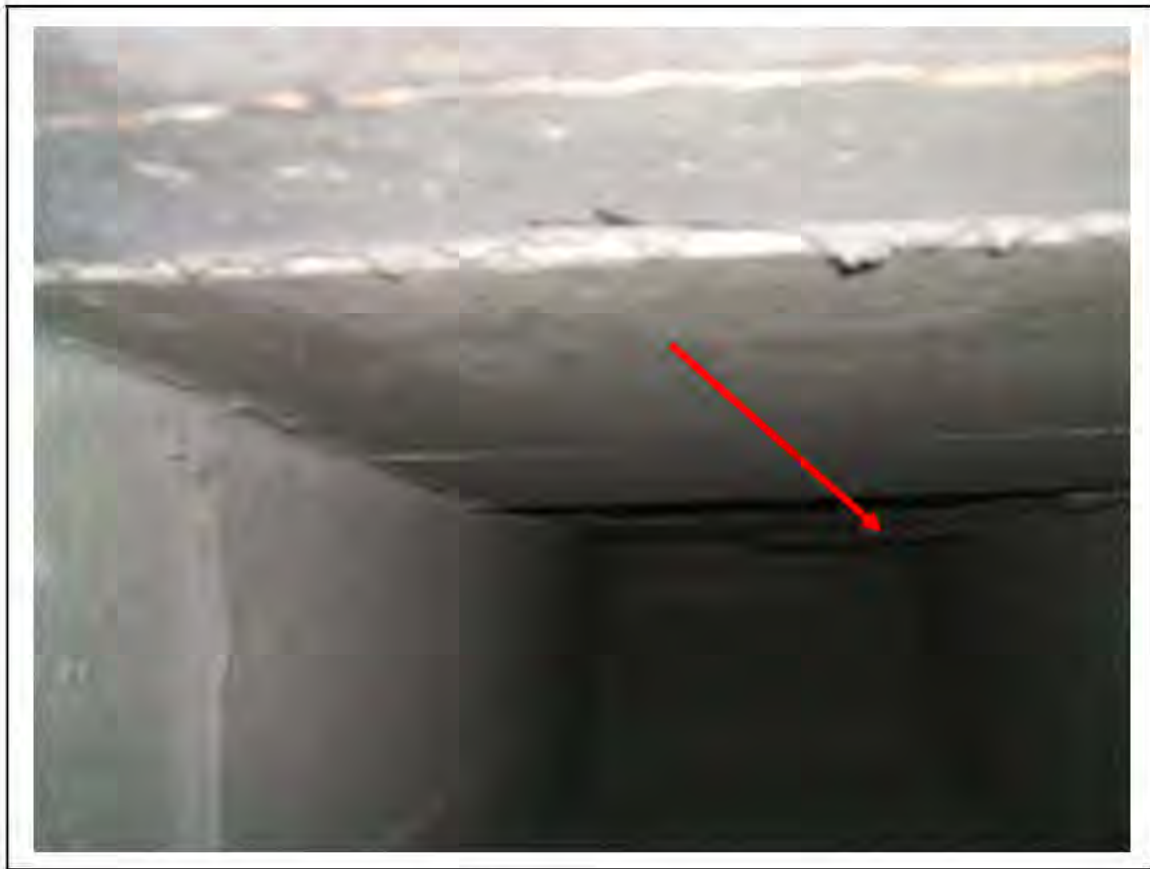
FIGURE 32: CONFIRMED ASBESTOS IN CEMENT BOARD SHUTTERING IN UMC , 2/151 - DESCRIPTION & RESULT OF ASSESSMENT (SAMPLE REF. 120445/150812/2)
