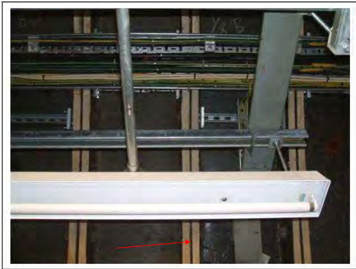
FIGURE 140: STRONGLY PRESUMED ASBESTOS IN TUNNEL RING CAULKING IN SWITCH ROOM E5, 3/662 - DESCRIPTION & RESULT OF ASSESSMENT (SAMPLE REF. SP1&2(1))
