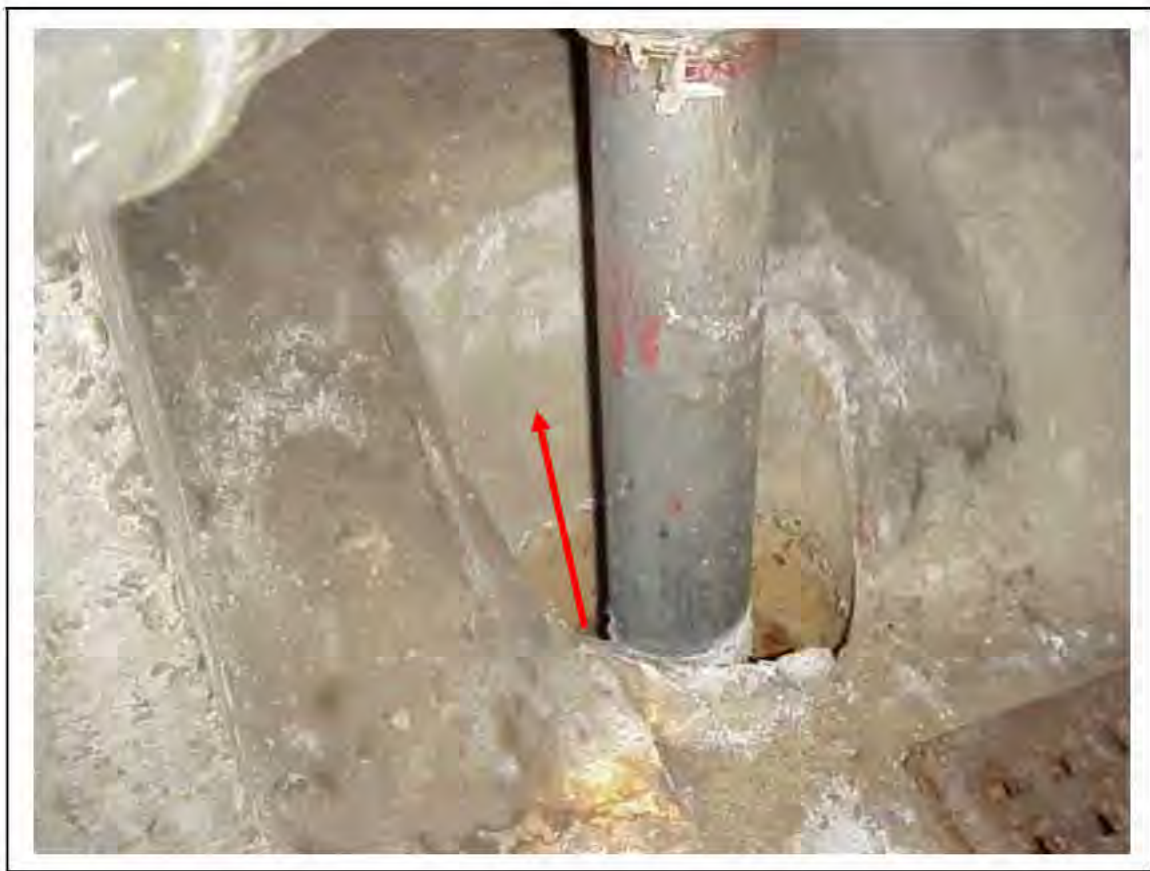
FIGURE 127: CONFIRMED ASBESTOS IN CABLE SLEEVE IN VICTORIA LINE, PLATFORM 2 INVERT, 3/262, 10M ON HALFWAY - DESCRIPTION & RESULT OF ASSESSMENT (SAMPLE REF. 034219/5)
