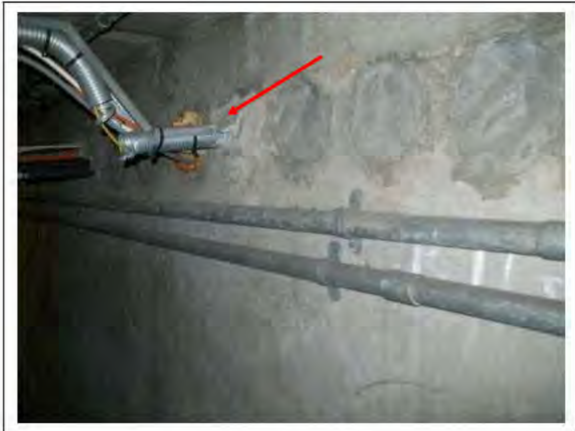
FIGURE 190: CONFIRMED ASBESTOS IN MID WALL DUCTS IN CABLE WAY, 3/787 - DESCRIPTION & RESULT OF ASSESSMENT (SAMPLE REF. 120445/190812/01)
