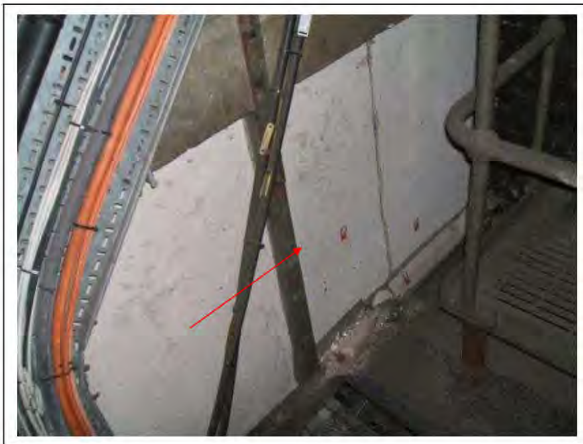
FIGURE 193: PRESUMED ASBESTOS IN RESIDUES BEHIND SUPALUX TO BEAM S10 IN VENT SHAFT , 3/902 - DESCRIPTION & RESULT OF ASSESSMENT (SAMPLE REF. P1&2(58))
