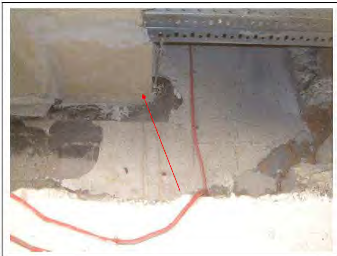
FIGURE 40: PRESUMED ASBESTOS IN BEAM VERMICULITE CLAD IN PASSAGE , 2/238 - DESCRIPTION & RESULT OF ASSESSMENT (SAMPLE REF. P1&2(27))
