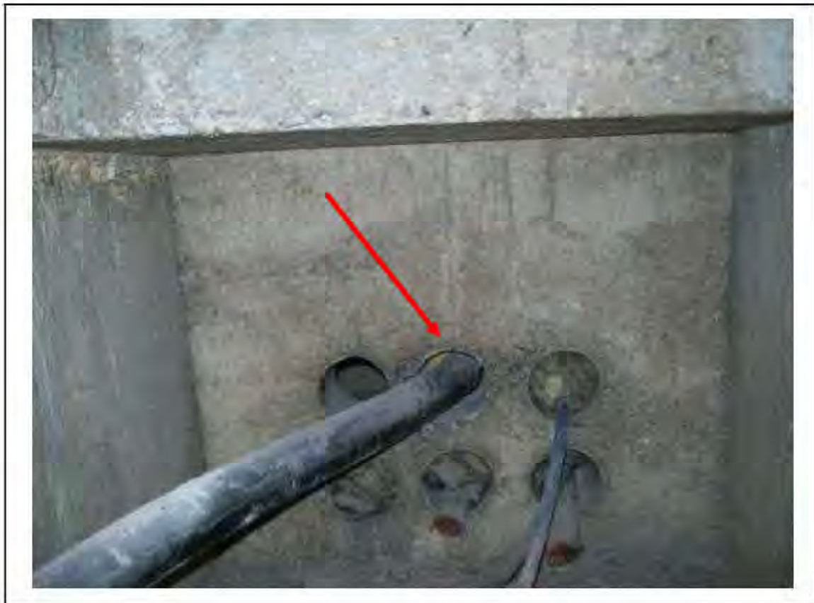
FIGURE 71: KNOWN ASBESTOS IN DUCTS IN CABLE PIT IN VENT ACCESS , 2/953 - DESCRIPTION & RESULT OF ASSESSMENT (SAMPLE REF. K1(7) PREVIOUS SAMPLE ECS78286)
