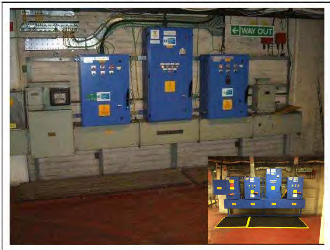
FIGURE 22: PRESUMED ASBESTOS IN BUS BAR BOX IN UMC, 2/151 - DESCRIPTION & RESULT OF ASSESSMENT (SAMPLE REF. P1(2))
