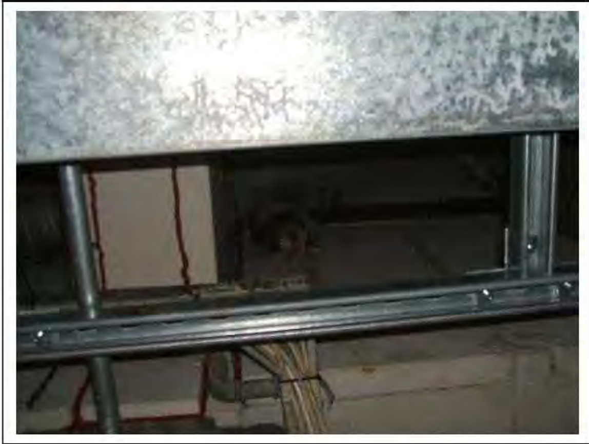
FIGURE 17: PRESUMED ASBESTOS IN RESIDUES WITHIN CONCRETE BY REDUNDANT SOIL PIPE THROUGH CEILING IN UMC ACCESS , 2/151 - DESCRIPTION & RESULT OF ASSESSMENT (SAMPLE REF. P1&2(16))
