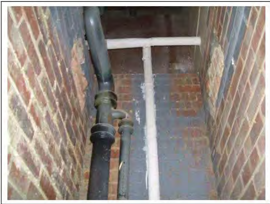
FIGURE 37: PRESUMED ASBESTOS IN RESIDUES IN WALL CAVITY IN RISER TO END CORRIDOR , 2/237 - DESCRIPTION & RESULT OF ASSESSMENT (SAMPLE REF. P1&2(24))
