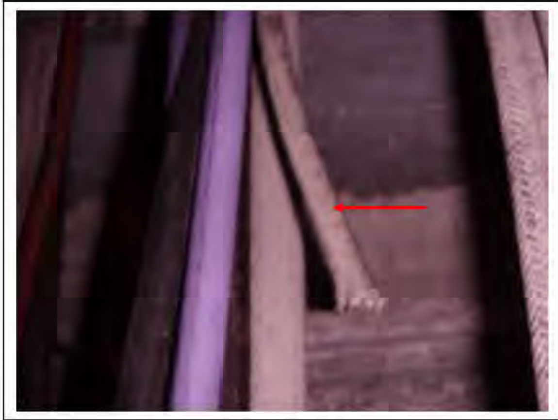
FIGURE 110: CONFIRMED ASBESTOS IN CABLE IN VICTORIA LINE, PLATFORM 1 INVERT, 3/261, DOWN HATCH NEAR 3/711 - DESCRIPTION & RESULT OF ASSESSMENT (SAMPLE REF. 034219/9)
