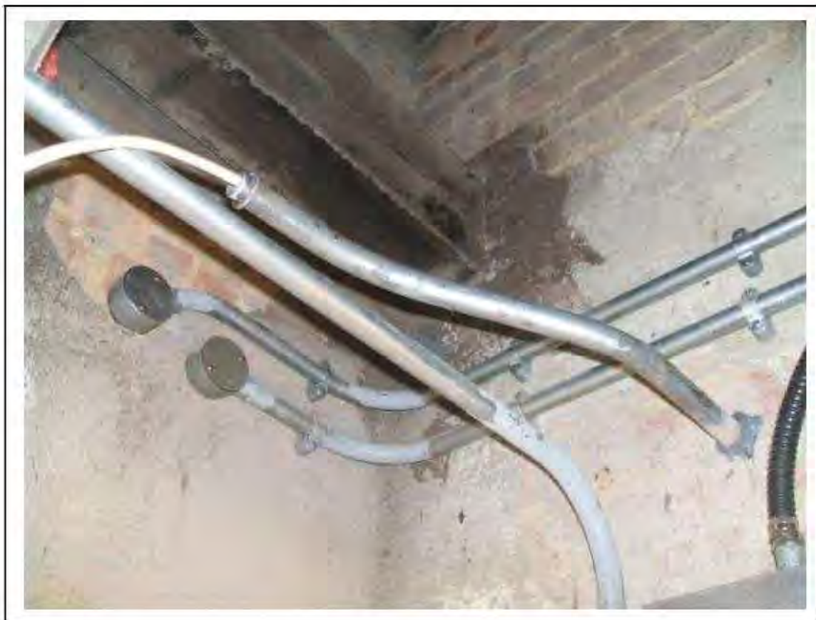
FIGURE 67: CONFIRMED ASBESTOS IN RESIDUE BELOW FOAM IN VENT ACCESS , 2/953 - DESCRIPTION & RESULT OF ASSESSMENT (SAMPLE REF. 120445/150812/04)
