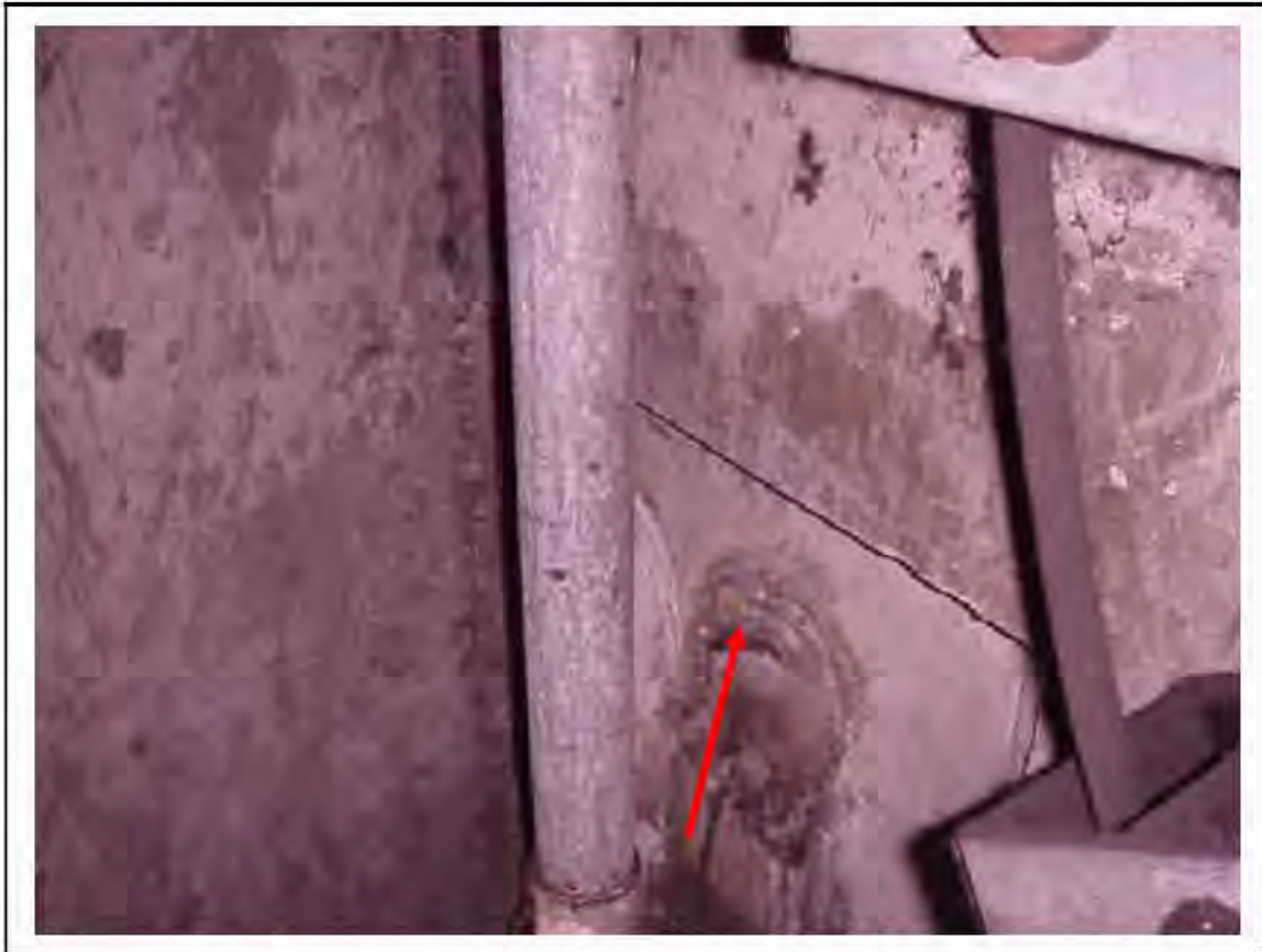
FIGURE 107: CONFIRMED ASBESTOS IN CABLE SLEEVES IN VICTORIA LINE, PLATFORM 1 INVERT, 3/261, DOWN HATCH NEAR 3/711 - DESCRIPTION & RESULT OF ASSESSMENT (SAMPLE REF. 034219/8)
