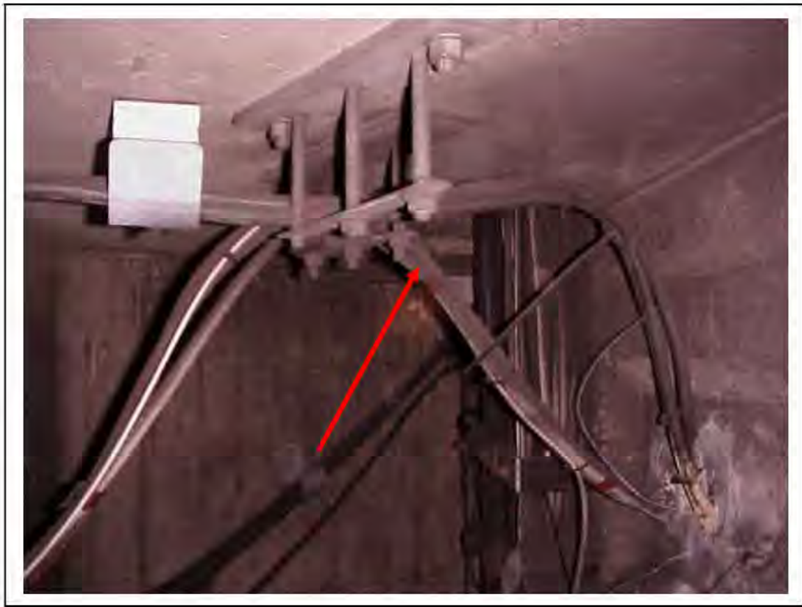
FIGURE 132: KNOWN ASBESTOS IN CABLES IN VICTORIA LINE, PLATFORM 2 INVERT, 3/262, OTHER END 3/706 - DESCRIPTION & RESULT OF ASSESSMENT (SAMPLE REF. K1(33))
