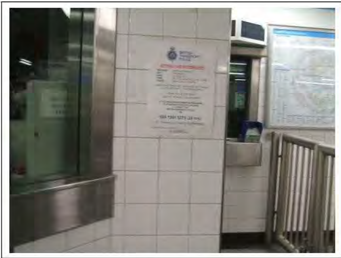
FIGURE 11: PRESUMED ASBESTOS IN RESIDUES WITHIN CIRCULATION AREA, 2/071 - DESCRIPTION & RESULT OF ASSESSMENT (SAMPLE REF. P1&2(11))
