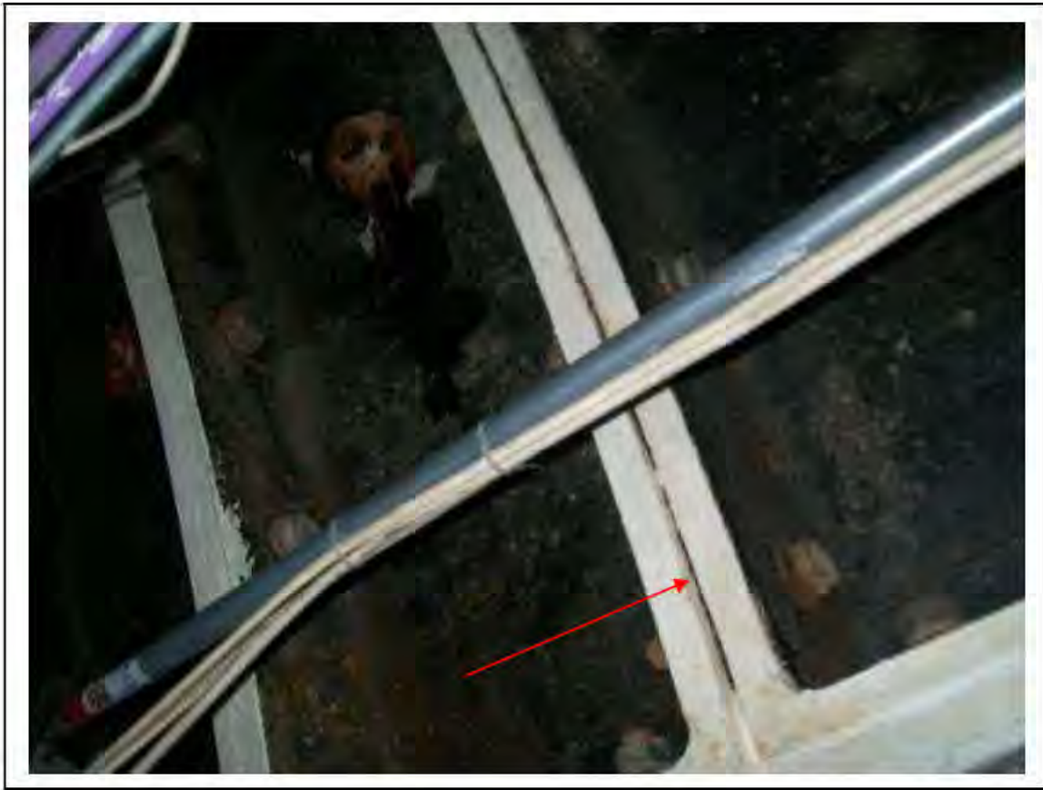
FIGURE 137: CONFIRMED ASBESTOS IN CAULKING IN LADIES LOBBY , 3/413 - DESCRIPTION & RESULT OF ASSESSMENT (SAMPLE REF. SAME AS 120445/150812/03)
