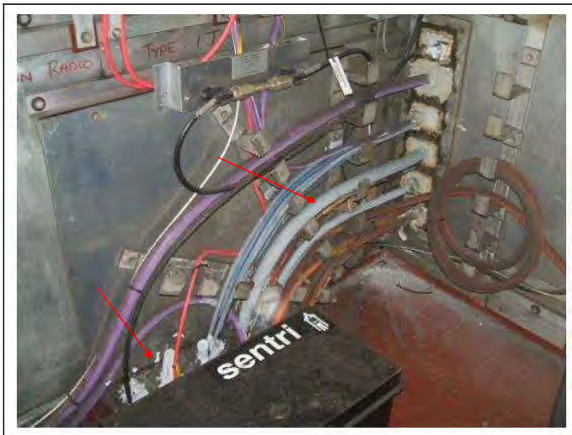
FIGURE 148: KNOWN ASBESTOS IN BRAIDED CABLES IN IMR (CORRIDOR FROM PLATFORM 1), 3/706 - DESCRIPTION & RESULT OF ASSESSMENT (SAMPLE REF. K1(36))
