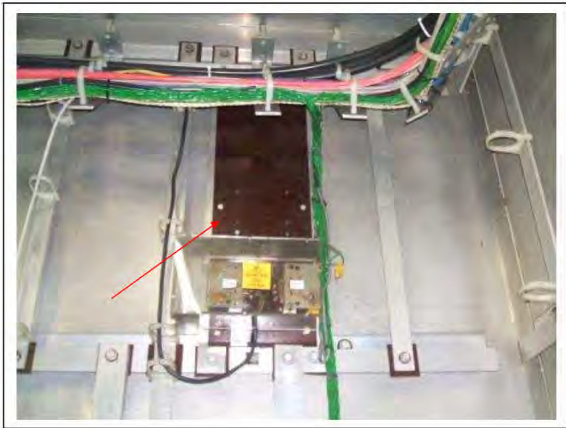
FIGURE 170: STRONGLY PRESUMED ASBESTOS IN SILUMINITE PANEL IN RELAY ROOM , 3/712 - DESCRIPTION & RESULT OF ASSESSMENT (SAMPLE REF. SP1(19))
