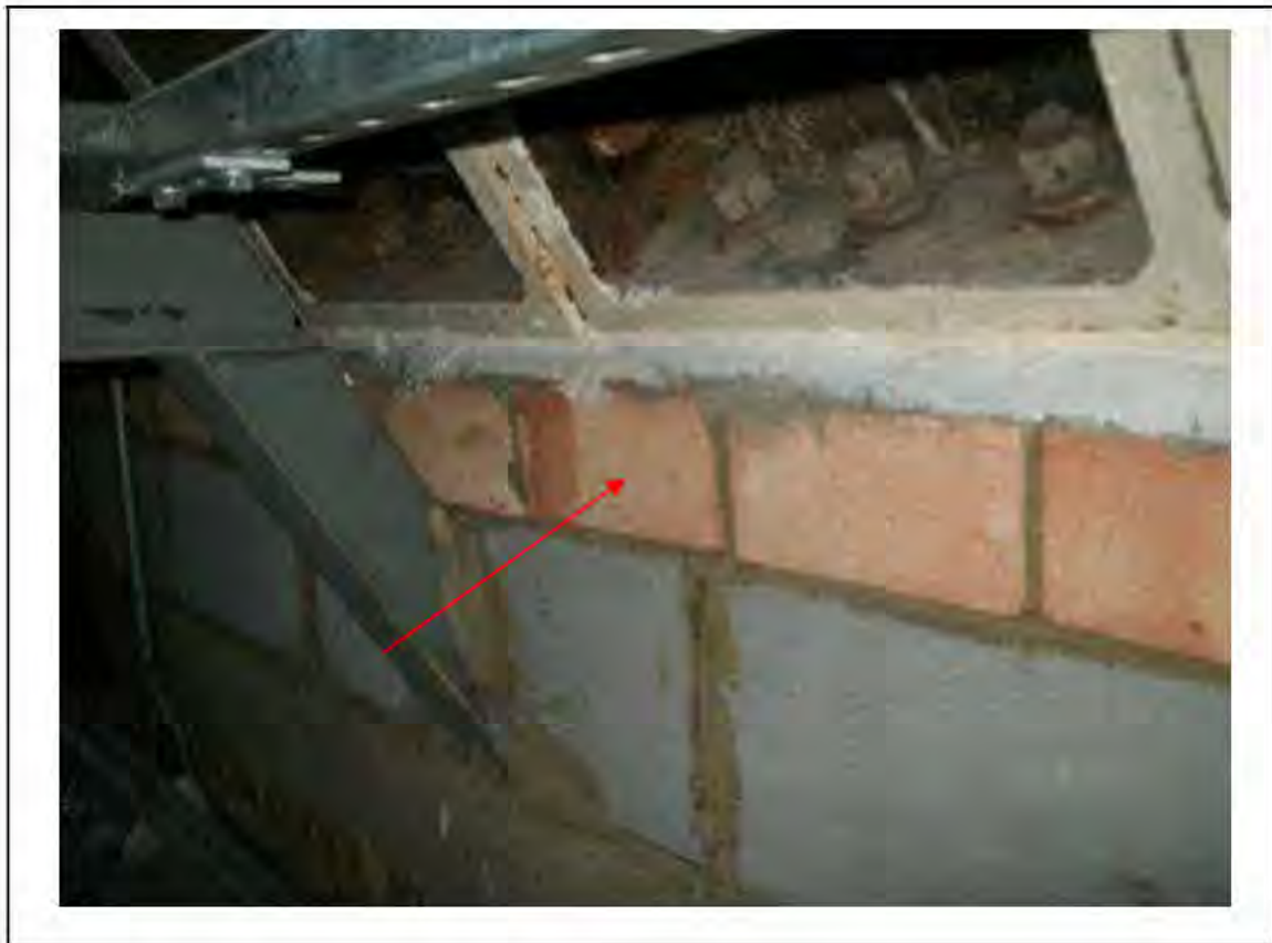
FIGURE 182: KNOWN ASBESTOS IN CELLACTITE, METAL CORRUGATED SHEETS IN OFFICE , 3/756 - DESCRIPTION & RESULT OF ASSESSMENT (SAMPLE REF. K1(46))
