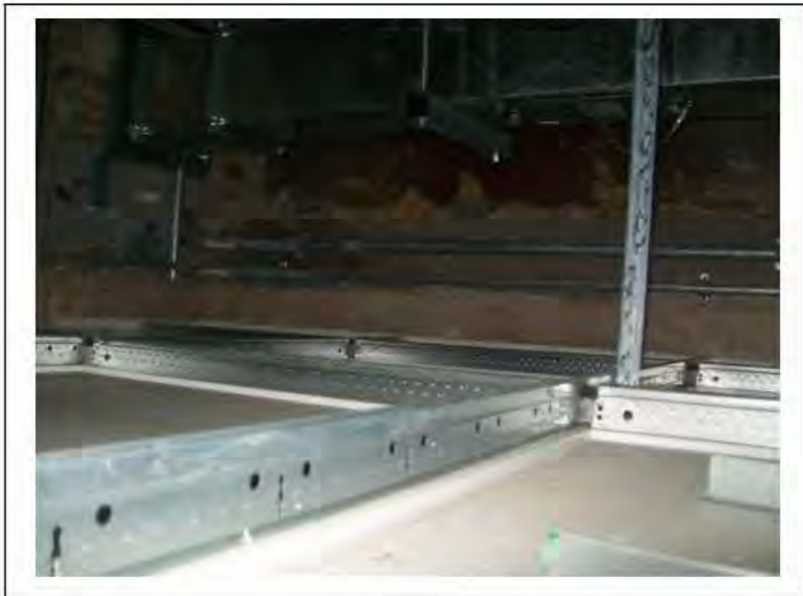
FIGURE 46: PRESUMED ASBESTOS IN RESIDUES WITHIN CALL CAVITY IN MESS ROOM / LOCKER ROOM, 2/281 - DESCRIPTION & RESULT OF ASSESSMENT (SAMPLE REF. P1&2(33))
