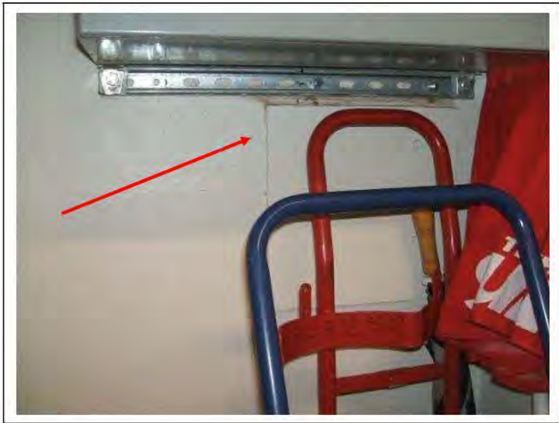
FIGURE 38: PRESUMED ASBESTOS BEHIND RENDER ON BRICK WALL IN PASSAGE , 2/238 - DESCRIPTION & RESULT OF ASSESSMENT (SAMPLE REF. P1&2(25))
