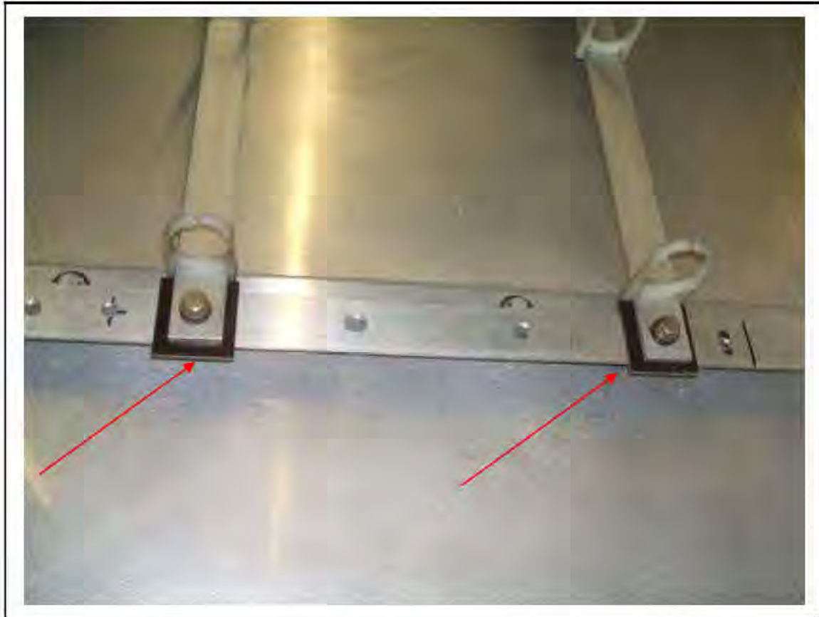
FIGURE 164: STRONGLY PRESUMED ASBESTOS IN SILUMINITE PACKING TO ALUMINIUM STRIP JOINTS IN RELAY ROOM , 3/711 - DESCRIPTION & RESULT OF ASSESSMENT (SAMPLE REF. SP1(15))
