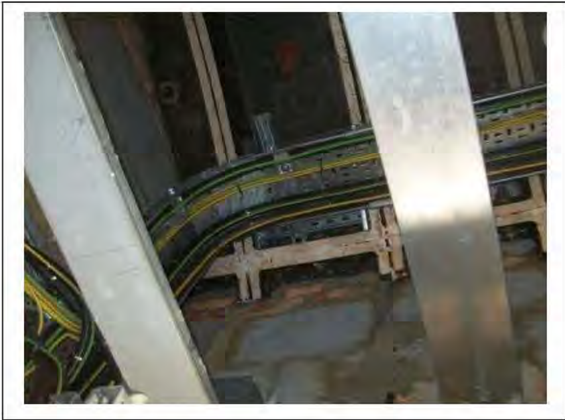
FIGURE 136: KNOWN ASBESTOS IN CAULKING IN SWITCH ROOM E10 , 3/412 - DESCRIPTION & RESULT OF ASSESSMENT (SAMPLE REF. SAME AS 120445/150812/03)
