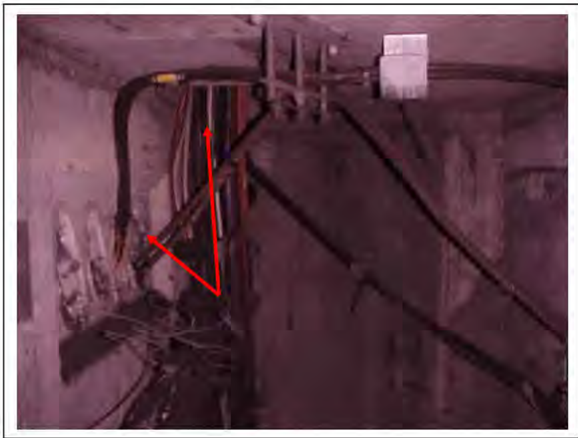
FIGURE 119: KNOWN ASBESTOS IN CABLES IN VICTORIA LINE, PLATFORM 1, 3/261 INVERT, OTHER END 3/706 - DESCRIPTION & RESULT OF ASSESSMENT (SAMPLE REF. K1(29))
