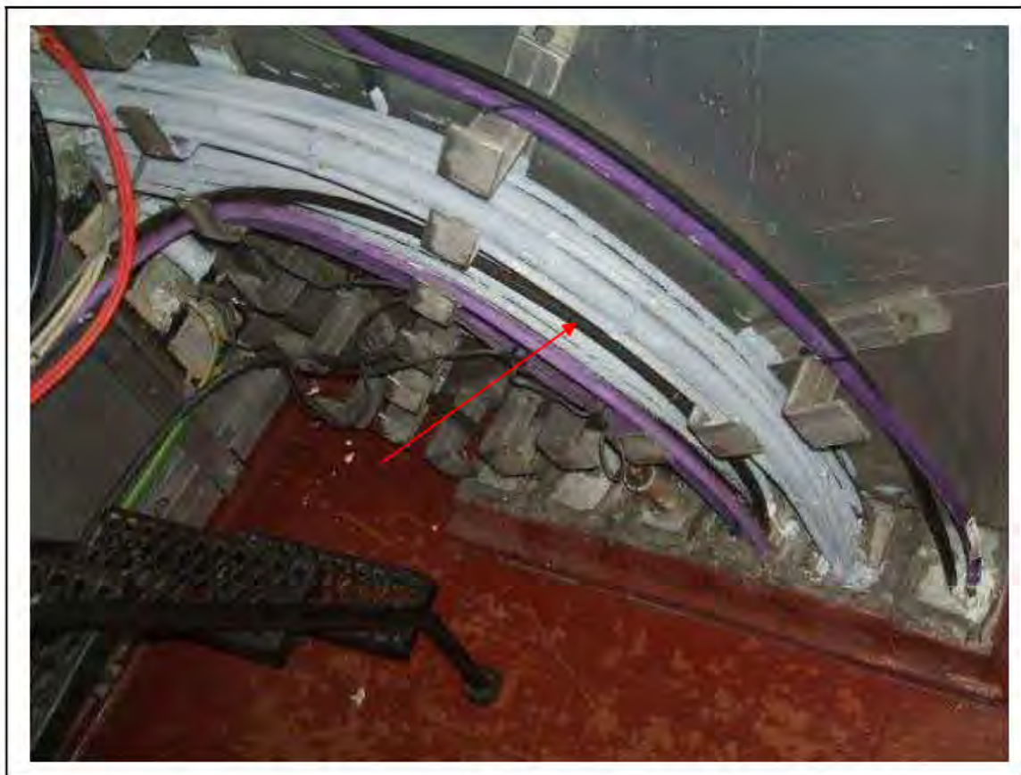
FIGURE 163: STRONGLY PRESUMED ASBESTOS IN BRAIDED CABLES IN RELAY ROOM , 3/711 - DESCRIPTION & RESULT OF ASSESSMENT (SAMPLE REF. SP1(14))
