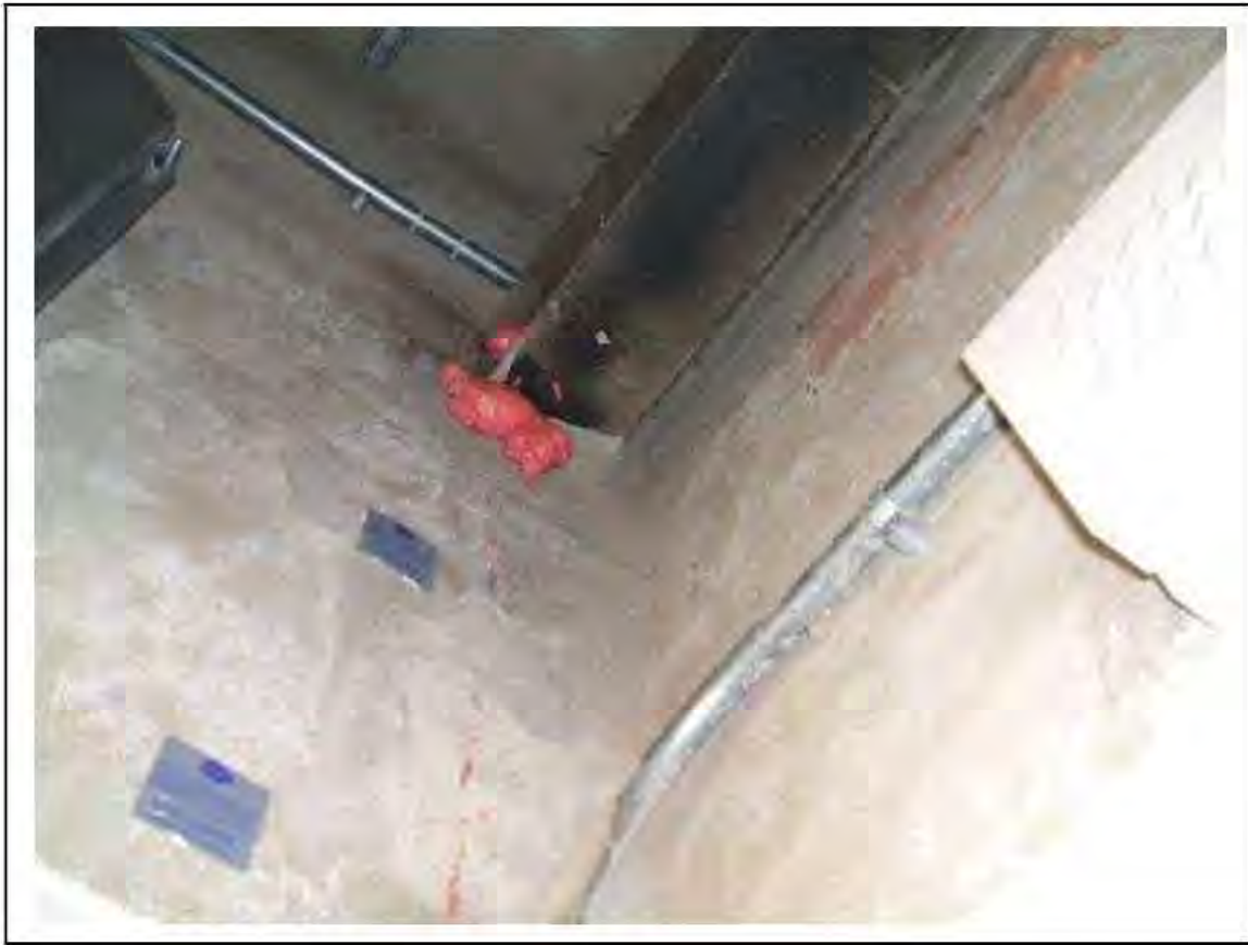
FIGURE 69: PRESUMED ASBESTOS IN RESIDUES IN VENT ACCESS , 2/953 - DESCRIPTION & RESULT OF ASSESSMENT (SAMPLE REF. P1&2(52))
