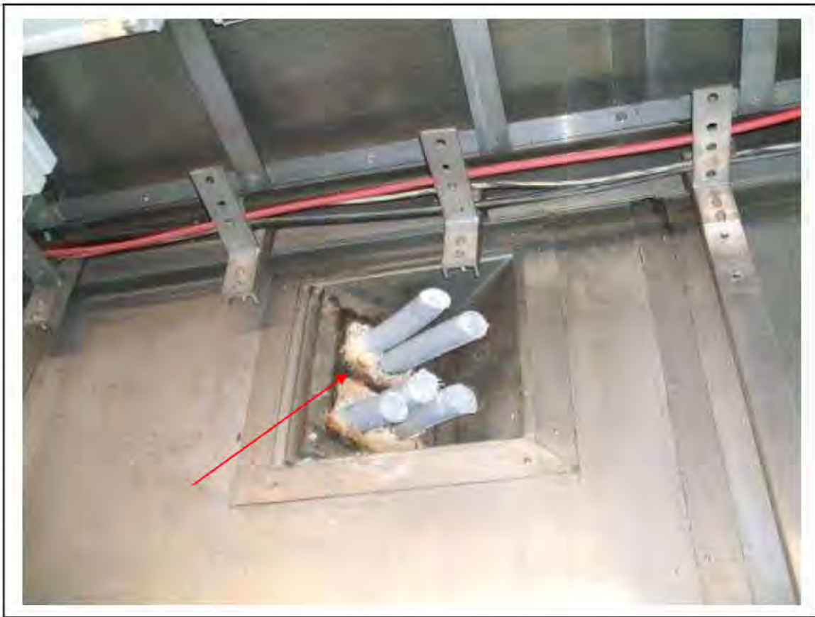
FIGURE 157: KNOWN ASBESTOS IN BRAIDED CABLES IN IMR (CORRIDOR TO PLATFORM 2), 3/706 - DESCRIPTION & RESULT OF ASSESSMENT (SAMPLE REF. K1(40))
