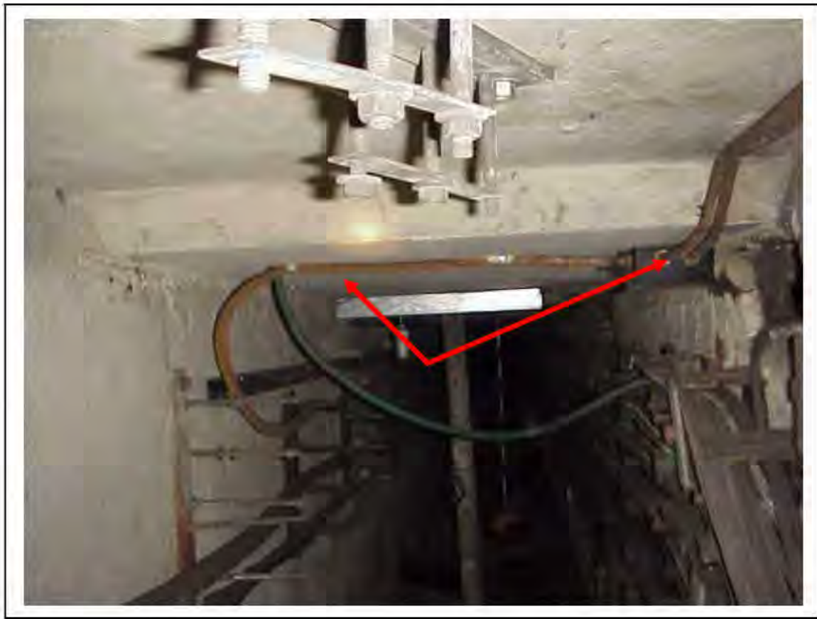
FIGURE 124: KNOWN ASBESTOS IN CABLES IN VICTORIA LINE, PLATFORM 2 INVERT, 3/262, DOWN HATCH NEAR 3/712 - DESCRIPTION & RESULT OF ASSESSMENT (SAMPLE REF. K1(31))
