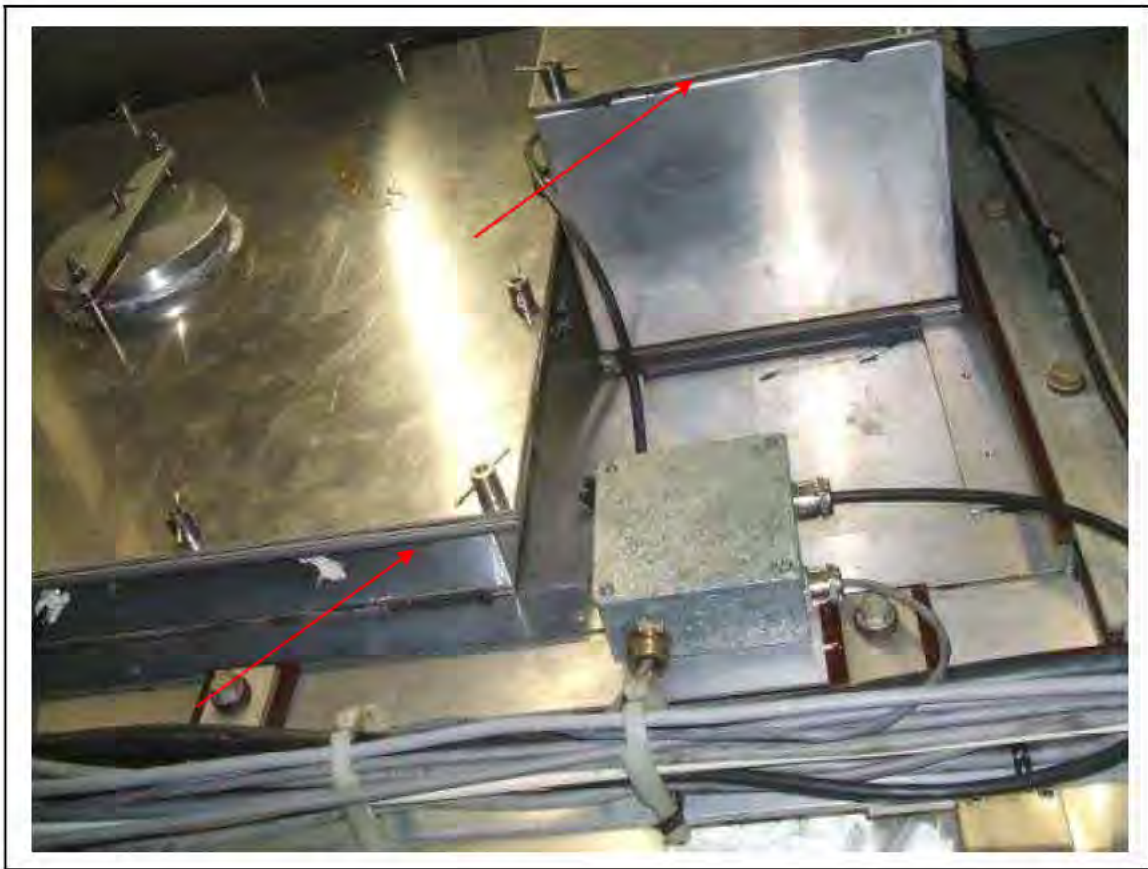
FIGURE 166: STRONGLY PRESUMED ASBESTOS IN PACKING IN RELAY ROOM , 3/711 - DESCRIPTION & RESULT OF ASSESSMENT (SAMPLE REF. SP1(17))
