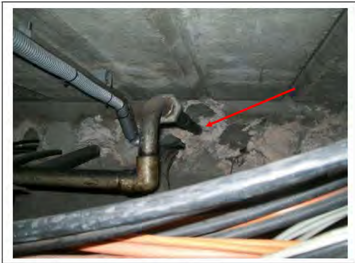
FIGURE 86: CONFIRMED ASBESTOS IN CABLE FLOOR DUCTS IN PASSAGE FLOOR DUCTS, 3/202 - DESCRIPTION & RESULT OF ASSESSMENT (SAMPLE REF. SAME AS 120445/190812/01)
