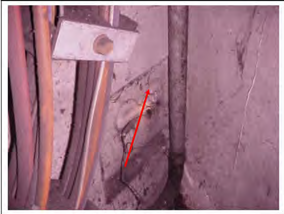
FIGURE 117: CONFIRMED ASBESTOS IN CABLE SLEEVES IN VICTORIA LINE, PLATFORM 1 INVERT, 3/261, OTHER END 3/706 - DESCRIPTION & RESULT OF ASSESSMENT (SAMPLE REF. SAME AS 034219/7,8,10)
