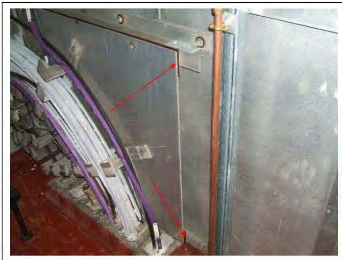
FIGURE 165: STRONGLY PRESUMED ASBESTOS IN SILUMINITE PACKING STRIPS IN RELAY ROOM , 3/711 - DESCRIPTION & RESULT OF ASSESSMENT (SAMPLE REF. SP1(16))
