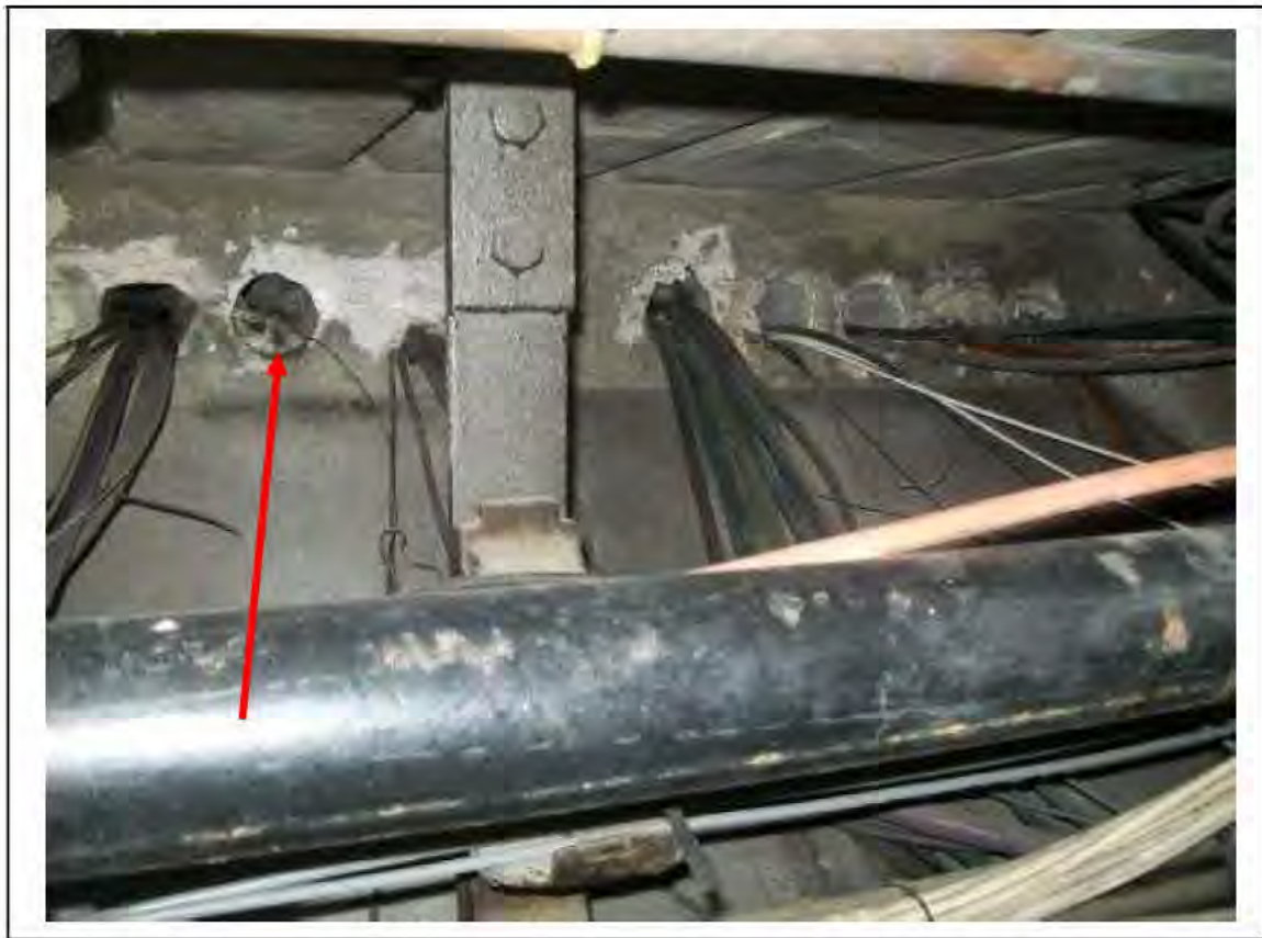
FIGURE 88: CONFIRMED ASBESTOS IN FLOOR CABLE DUCTS IN PASSAGE , 3/203 - DESCRIPTION & RESULT OF ASSESSMENT (SAMPLE REF. SAME AS 120445/190812/01)
