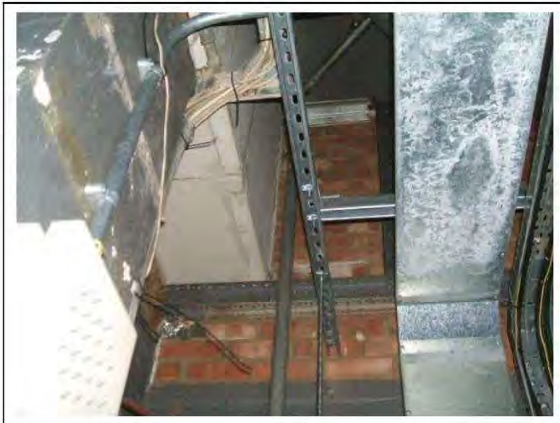
FIGURE 18: PRESUMED ASBESTOS IN RESIDUE BENEATH PAINT WHERE BEAM S10 PASSES INTO WALL IN UMC ACCESS , 2/151 - DESCRIPTION & RESULT OF ASSESSMENT (SAMPLE REF. P1&2(17))
