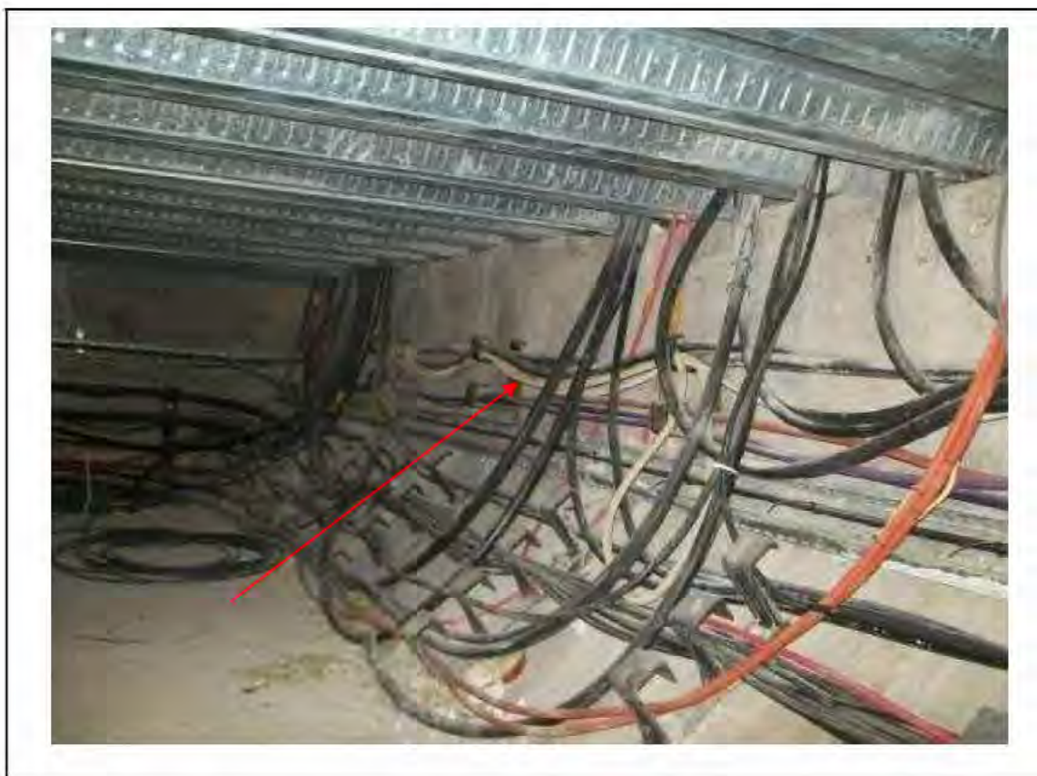
FIGURE 97: KNOWN ASBESTOS IN BRAIDED CABLE IN PASSAGE CABLE DUCT/TRENCH, 3/207 - DESCRIPTION & RESULT OF ASSESSMENT (SAMPLE REF. K1(21))
