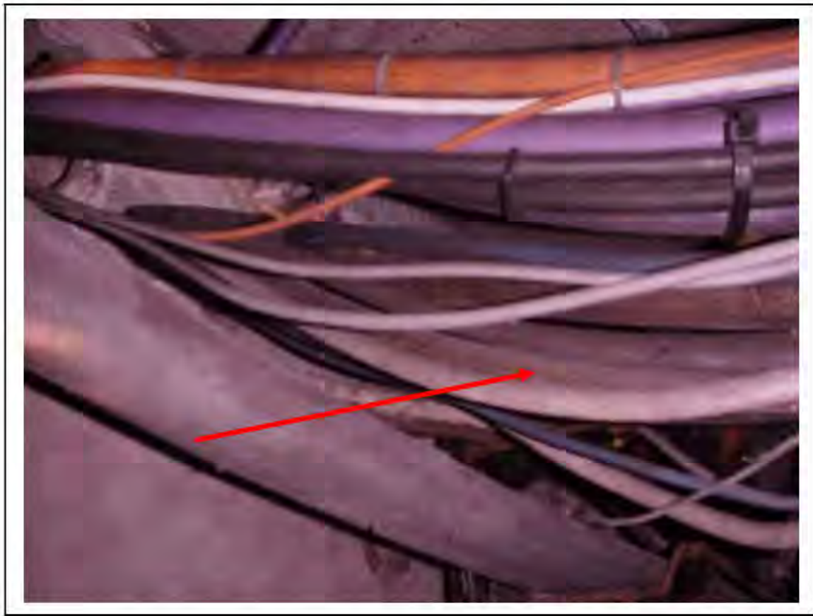
FIGURE 114: KNOWN ASBESTOS IN CABLES IN VICTORIA LINE, PLATFORM 1 INVERT, 3/261, 30M UP - DESCRIPTION & RESULT OF ASSESSMENT (SAMPLE REF. K1(28))
