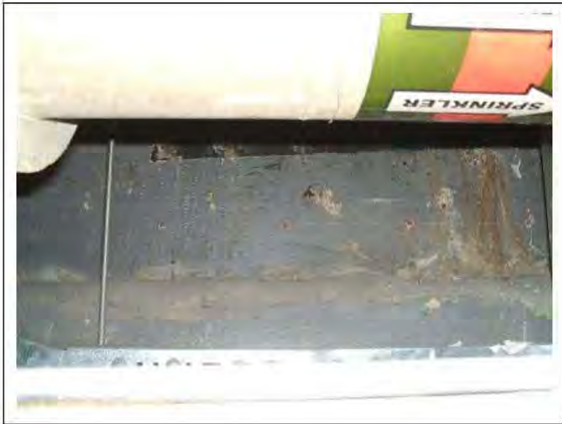
FIGURE 45: PRESUMED ASBESTOS IN FIBREBOARD CLAD BEAM OVER END OF 2/407 AND 2/669 IN PASSAGE , 2/238 - DESCRIPTION & RESULT OF ASSESSMENT (SAMPLE REF. P1&2(32))
