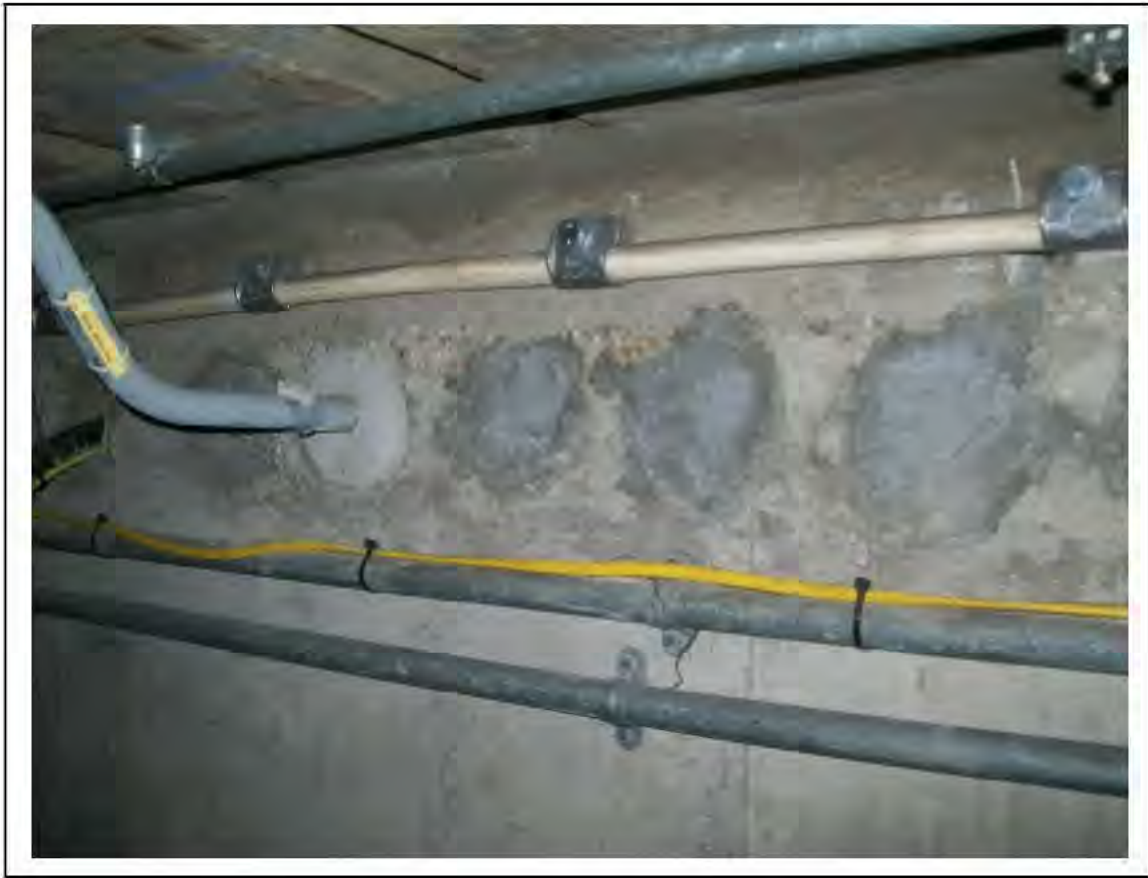
FIGURE 191: KNOWN ASBESTOS IN MID WALL DUCTS IN CABLE WAY, 3/787 - DESCRIPTION & RESULT OF ASSESSMENT (SAMPLE REF. SAME AS 120445/190812/01)
