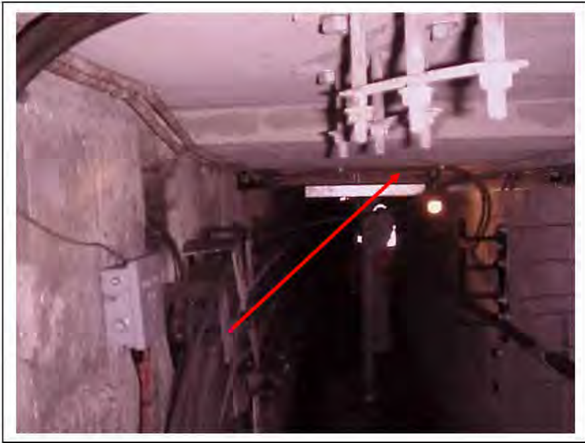
FIGURE 111: KNOWN ASBESTOS IN CABLE IN VICTORIA LINE, PLATFORM 1 INVERT, 3/261, DOWN HATCH NEAR 3/711 - DESCRIPTION & RESULT OF ASSESSMENT (SAMPLE REF. K1(26))
