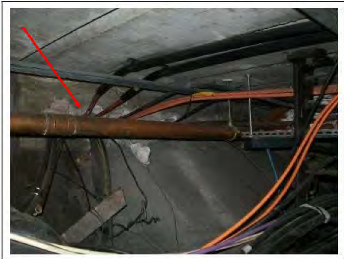
FIGURE 92: CONFIRMED ASBESTOS IN CABLE DUCTS IN PASSAGE FLOOR DUCTS, 3/206 - DESCRIPTION & RESULT OF ASSESSMENT (SAMPLE REF. SAME AS 120445/190812/01)
