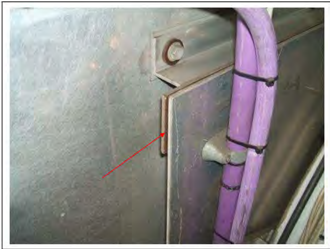
FIGURE 174: STRONGLY PRESUMED ASBESTOS IN SILUMINITE PACKING STRIPS IN RELAY ROOM , 3/712 - DESCRIPTION & RESULT OF ASSESSMENT (SAMPLE REF. SP1(23))
