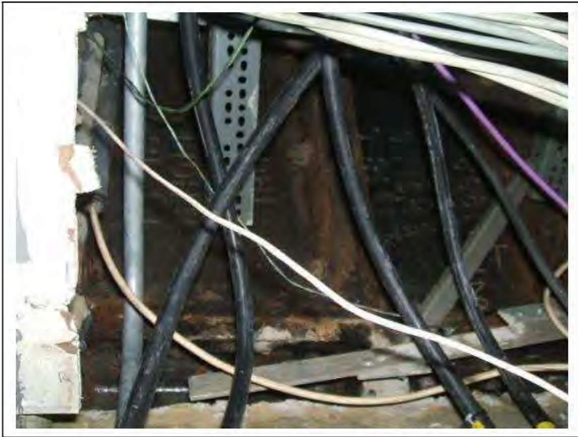
FIGURE 177: STRONGLY PRESUMED ASBESTOS IN TUNNEL RING JOINTS IN CER, 3/731 - DESCRIPTION & RESULT OF ASSESSMENT (SAMPLE REF. SP1&2(2))
