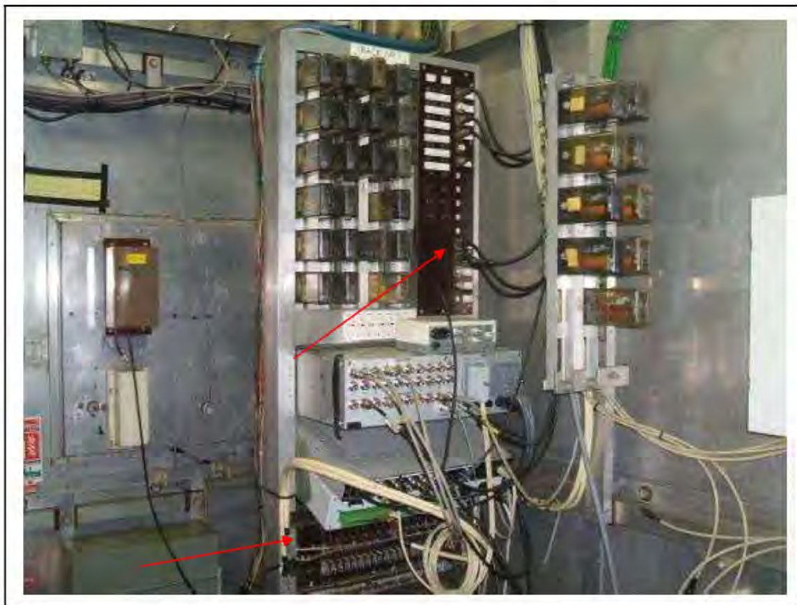
FIGURE 176: STRONGLY PRESUMED ASBESTOS IN SILUMINITE BOARDS IN RELAY ROOM , 3/712 - DESCRIPTION & RESULT OF ASSESSMENT (SAMPLE REF. SP1(25))
