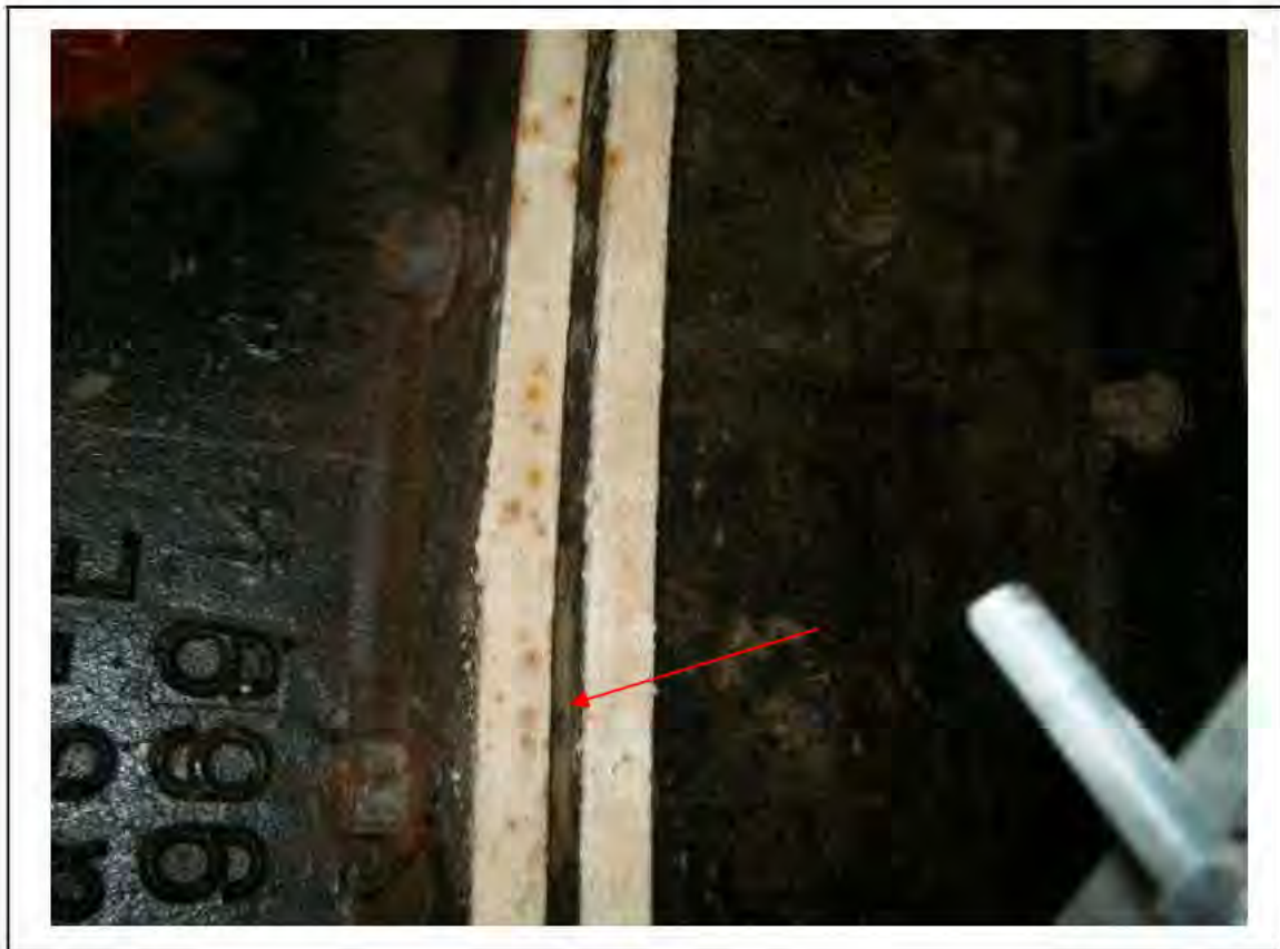
FIGURE 73: CONFIRMED ASBESTOS IN CAULKING TO TUNNEL RING JOINTS IN SWITCH ROOM E14, 3/047 - DESCRIPTION & RESULT OF ASSESSMENT (SAMPLE REF. AS 120445/150812/03)
