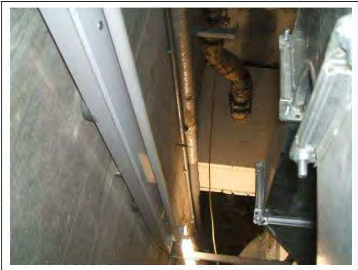
FIGURE 65: PRESUMED ASBESTOS IN RESIDUES WHERE BEAMS ENTER WALL IN SERVICE VOID , 2/902 - DESCRIPTION & RESULT OF ASSESSMENT (SAMPLE REF. P1&2(49))
