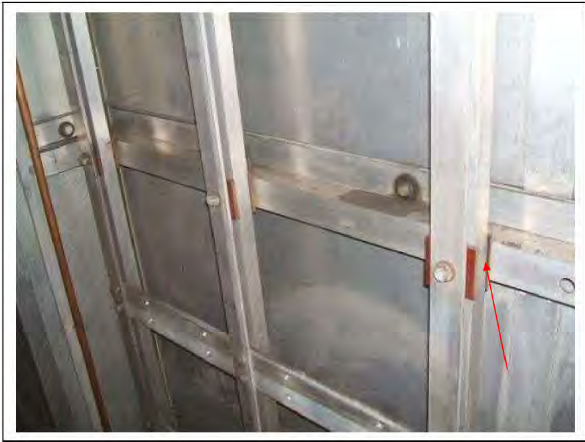
FIGURE 151: STRONGLY PRESUMED ASBESTOS IN SILUMINITE PACKING IN IMR , 3/706 - DESCRIPTION & RESULT OF ASSESSMENT (SAMPLE REF. SP1(8))
