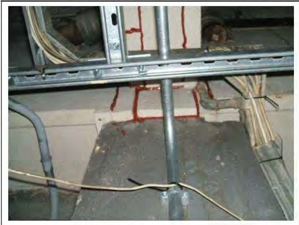
FIGURE 19: PRESUMED ASBESTOS IN RESIDUE REMAINING IN SMALL GAP BETWEEN BEAMS S9 AND S10 AND TOP OF WALL AND VOID OVER ESCALATOR IN UMC ACCESS , 2/151 - DESCRIPTION & RESULT OF ASSESSMENT (SAMPLE REF. P1&2(18))
