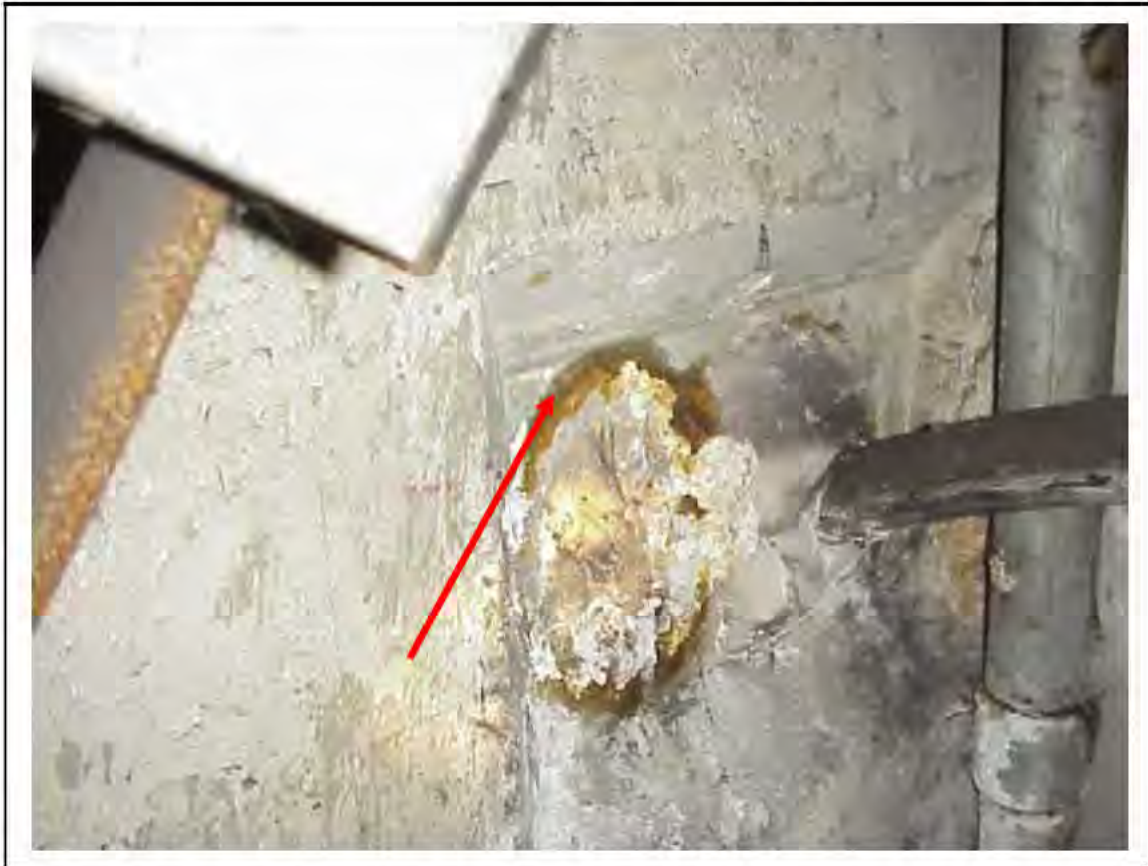
FIGURE 121: CONFIRMED ASBESTOS IN CABLE SLEEVES IN VICTORIA LINE, PLATFORM 2 INVERT, 3/262, DOWN HATCH NEAR 3/712 - DESCRIPTION & RESULT OF ASSESSMENT (SAMPLE REF. 034219/2)
