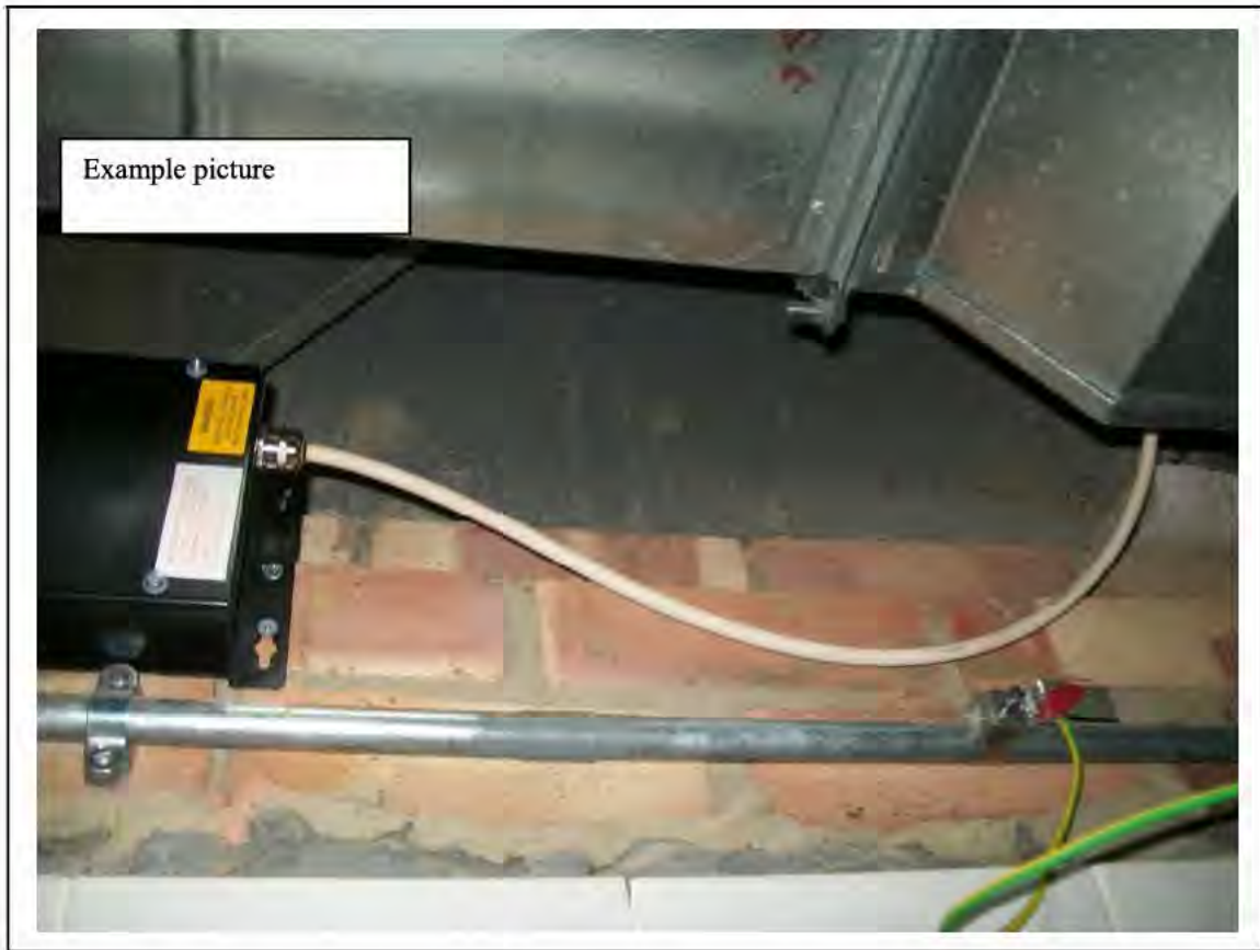
FIGURE 57: PRESUMED ASBESTOS IN RESIDUAL SPRAY INSULATION IN WALL CAVITY IN OFFICE , 2/418 - DESCRIPTION & RESULT OF ASSESSMENT (SAMPLE REF. P1&2(43))
