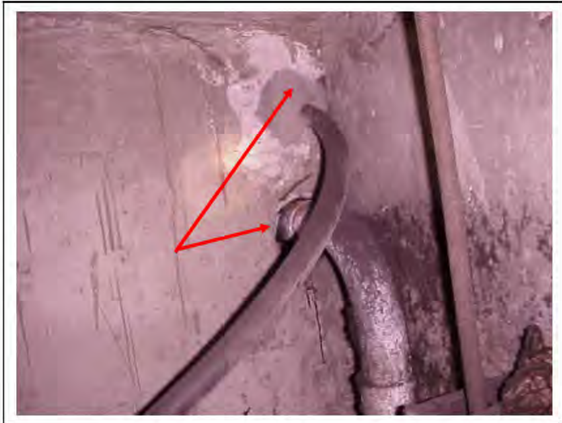
FIGURE 106: CONFIRMED ASBESTOS IN CABLE SLEEVES IN VICTORIA LINE, PLATFORM 1 INVERT, 3/261, DOWN HATCH NEAR 3/711 - DESCRIPTION & RESULT OF ASSESSMENT (SAMPLE REF. 034219/7)
