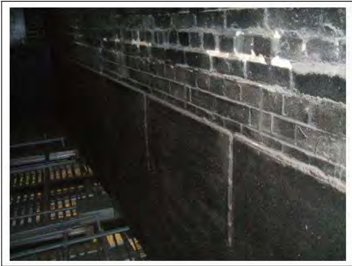
FIGURE 192: PRESUMED ASBESTOS BEHIND PANELS TO BEAM IN VENT SHAFT , 3/902 - DESCRIPTION & RESULT OF ASSESSMENT (SAMPLE REF. P1&2(57))
