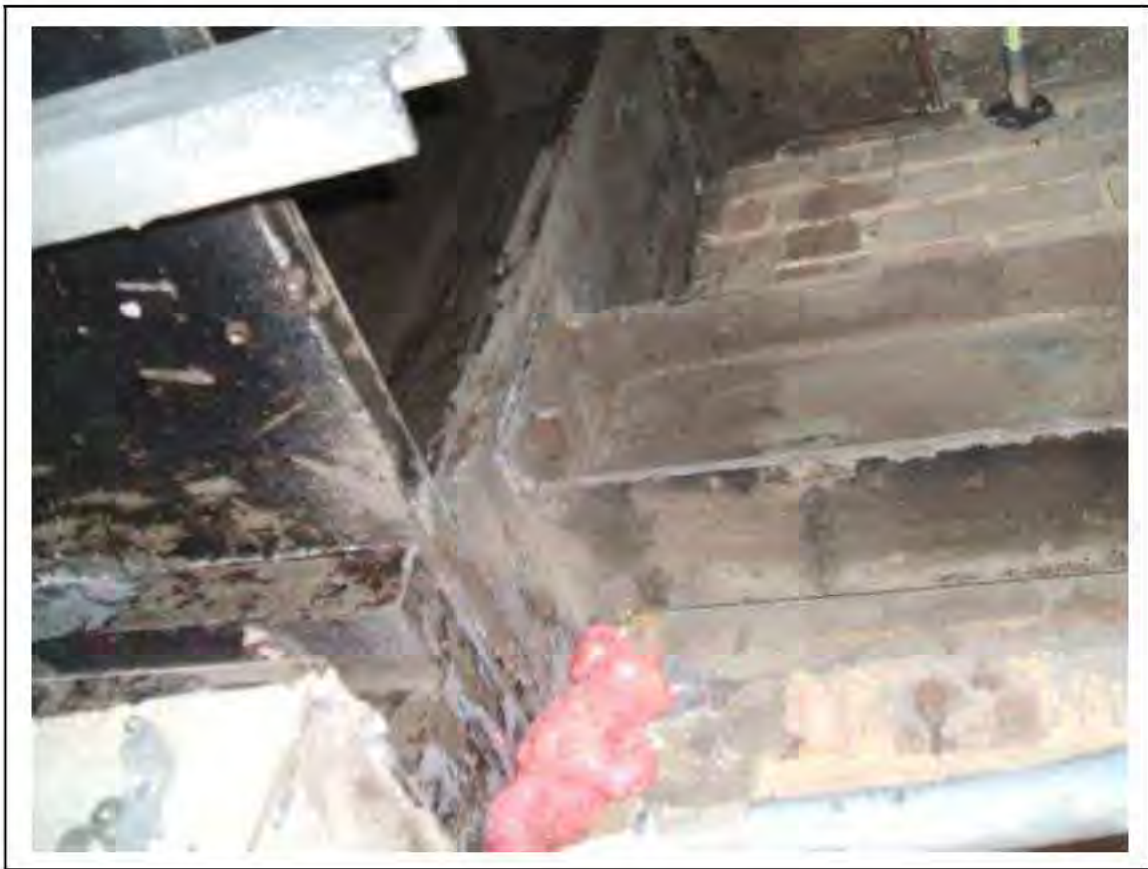
FIGURE 68: PRESUMED ASBESTOS IN RESIDUES IN VOID BY BEAM S12 IN VENT ACCESS , 2/953 - DESCRIPTION & RESULT OF ASSESSMENT (SAMPLE REF. P1&2(51))
