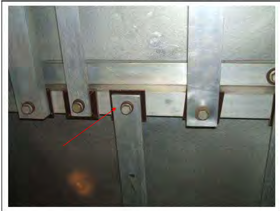
FIGURE 172: STRONGLY PRESUMED ASBESTOS IN PACKING TO ALUMINIUM STRIP JOINTS (SILUMINITE) IN RELAY ROOM , 3/712 - DESCRIPTION & RESULT OF ASSESSMENT (SAMPLE REF. SP1(21))
