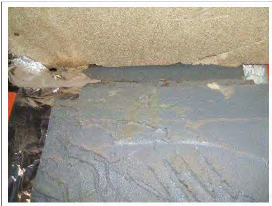
FIGURE 43: PRESUMED ASBESTOS IN BEAM FIBREBOARD CLAD OVER 2/661, 2662 AND IN PASSAGE , 2/238 - DESCRIPTION & RESULT OF ASSESSMENT (SAMPLE REF. P1&2(30))
