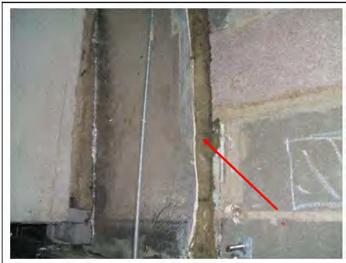
FIGURE 3: PRESUMED ASBESTOS IN RESIDUES BEHIND OLD VERMICULITE CLADDING N TICKET OFFICE CORRIDOR, 2/011 - DESCRIPTION & RESULT OF ASSESSMENT (SAMPLE REF. P1&2(3))
