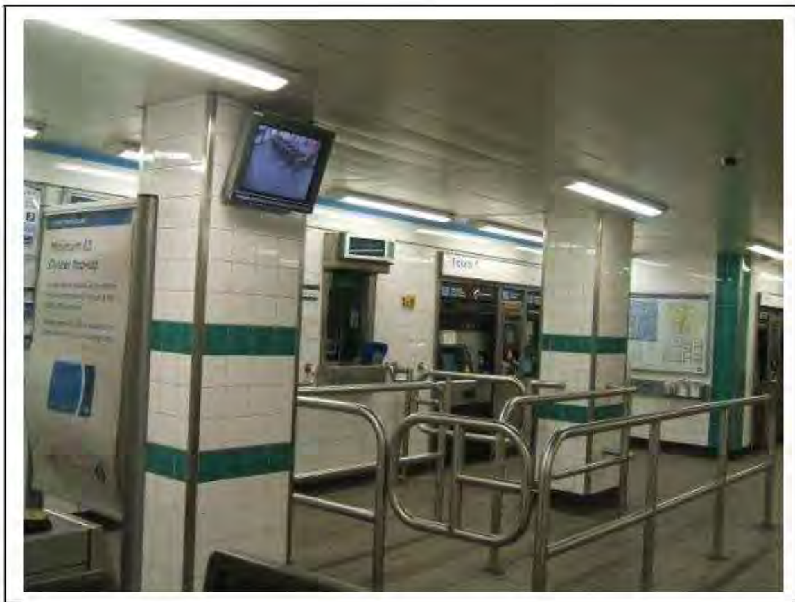
FIGURE 2: PRESUMED ASBESTOS ABOVE FALSE CEILING IN TICKET HALL, 2/001 - DESCRIPTION & RESULT OF ASSESSMENT (SAMPLE REF. P1&2(2))
