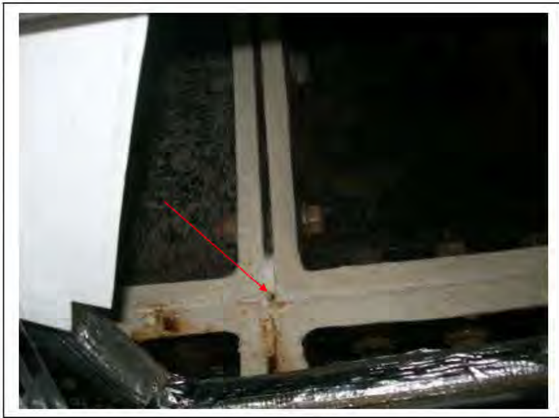
FIGURE 138: CONFIRMED ASBESTOS IN CAULKING IN LADIES W/C, 3/417 - DESCRIPTION & RESULT OF ASSESSMENT (SAMPLE REF. SAME AS 120445/150812/03)
