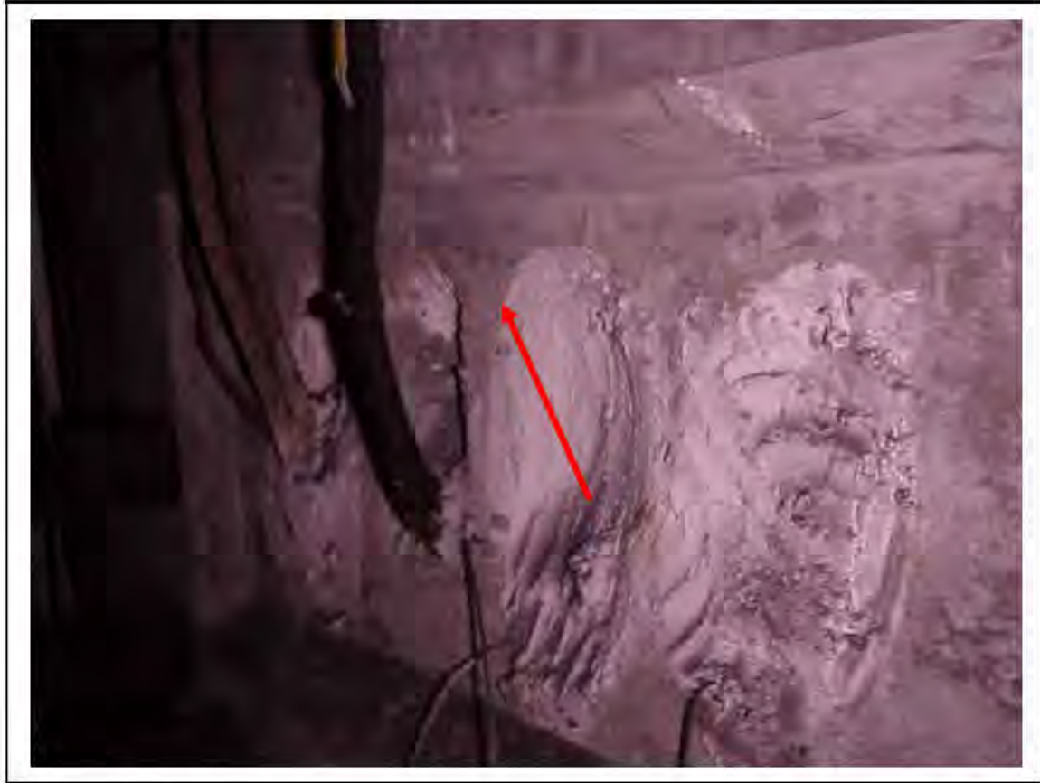
FIGURE 108: CONFIRMED ASBESTOS IN CABLE SLEEVES IN VICTORIA LINE, PLATFORM 1 INVERT, 3/261, DOWN HATCH NEAR 3/711 - DESCRIPTION & RESULT OF ASSESSMENT (SAMPLE REF. AS 034219/7&8)
