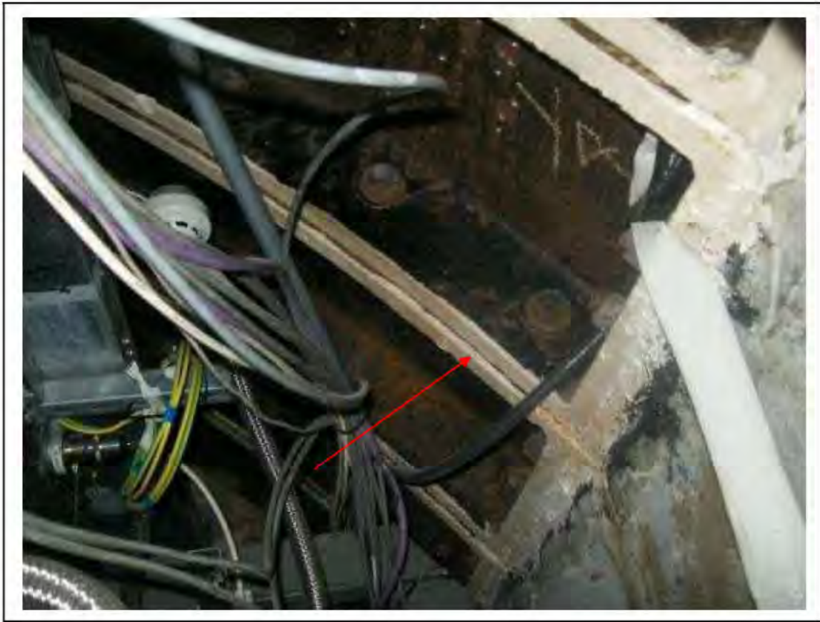
FIGURE 183: CONFIRMED ASBESTOS IN CAULKING IN PUMP ROOM, 3/771 - DESCRIPTION & RESULT OF ASSESSMENT (SAMPLE REF. SAME AS 120445/150812/03)
