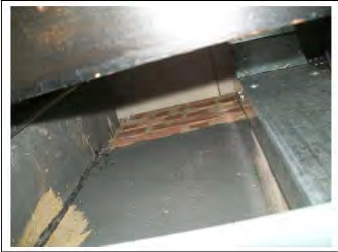
FIGURE 59: PRESUMED ASBESTOS IN POSSIBLE RESIDUES ABOVE SUPALUX PANEL TO CEILING IN SWITCH ROOM , 2/663 - DESCRIPTION & RESULT OF ASSESSMENT (SAMPLE REF. P1&2(44))
