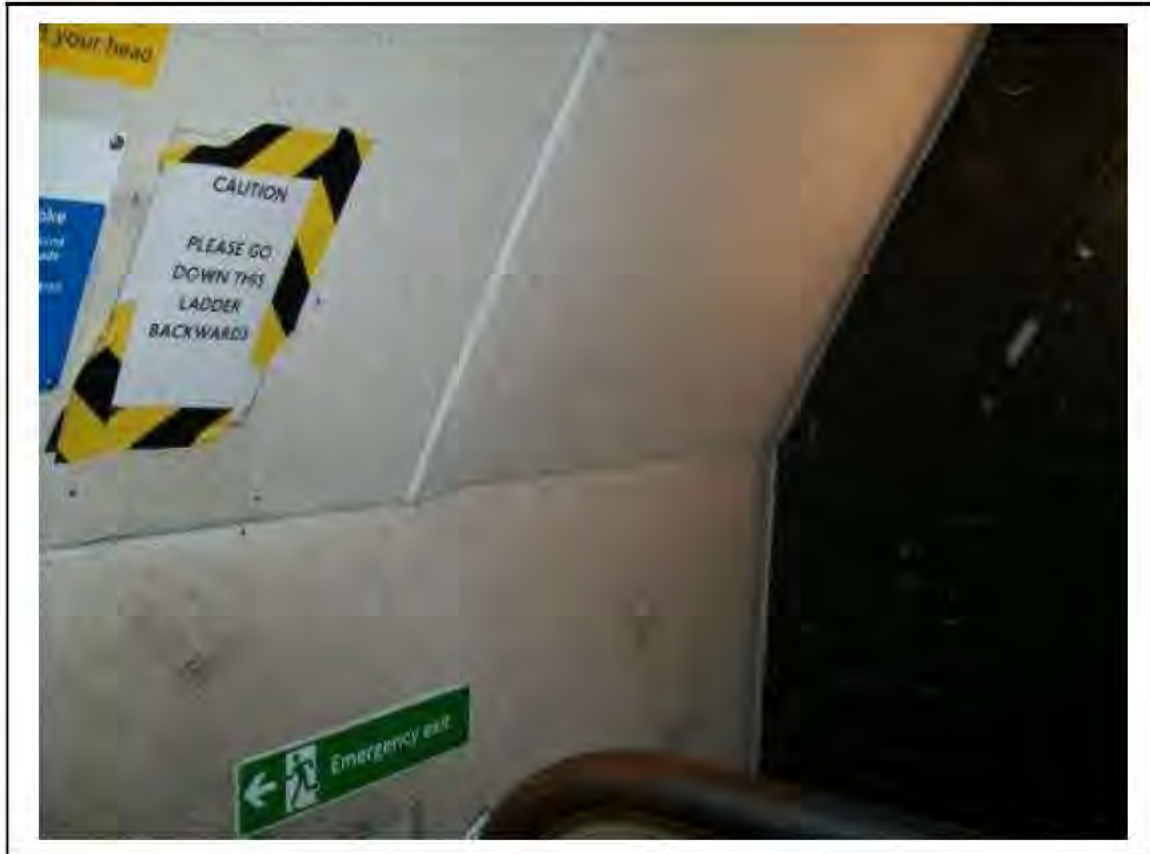
FIGURE 82: PRESUMED ASBESTOS BEHIND SUPALUX, POSSIBLE CELLACTITE AND CAULKING BEHIND IN LMC ACCESS, 3/161 - DESCRIPTION & RESULT OF ASSESSMENT (SAMPLE REF. P1&2(54))
