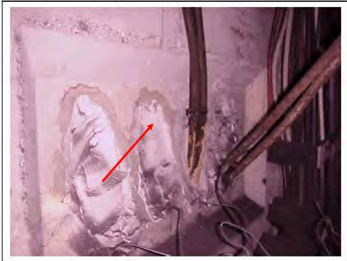
FIGURE 118: CONFIRMED ASBESTOS IN CABLE SLEEVES IN VICTORIA LINE, PLATFORM 1 INVERT, 3/261, OTHER END 3/706 - DESCRIPTION & RESULT OF ASSESSMENT (SAMPLE REF. SAME AS 034219/7,8,10)
