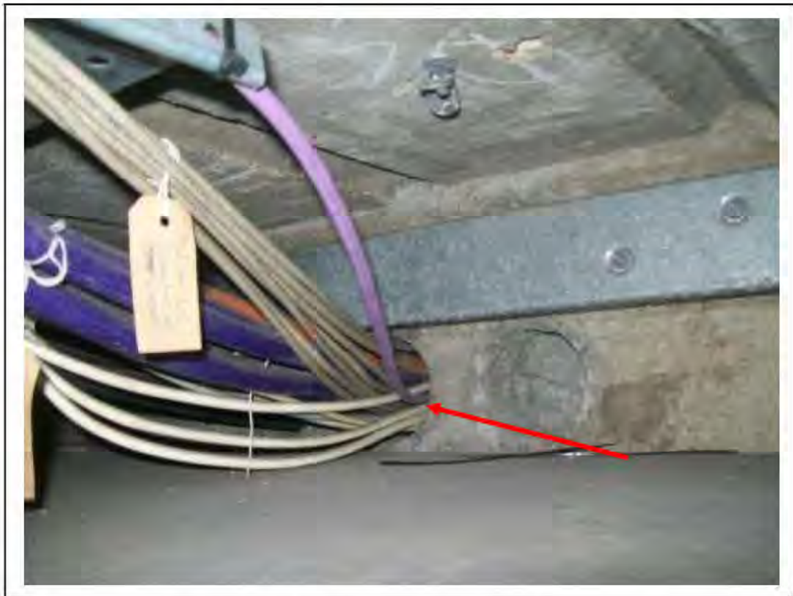
FIGURE 186: CONFIRMED ASBESTOS IN DUCT TO MID WALL IN CABLE SHAFT, 3/786 - DESCRIPTION & RESULT OF ASSESSMENT (SAMPLE REF. SAME AS 120445/190812/01)
