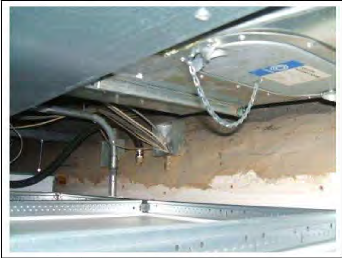
FIGURE 5: PRESUMED ASBESTOS - POSSIBLE RESIDUES BEHIND FALSE WALL TO EXTERNAL SIDE IN TICKET OFFICE, 2/011 - DESCRIPTION & RESULT OF ASSESSMENT (SAMPLE REF. P1&2(5))
