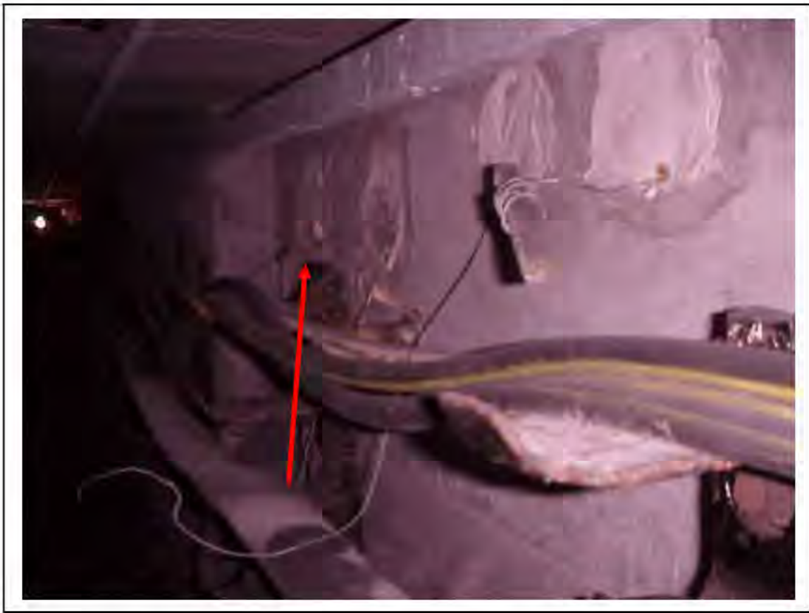
FIGURE 112: PRESUMED ASBESTOS IN CABLE SLEEVES IN VICTORIA LINE, PLATFORM 1 INVERT, 3/261, 30M UP - DESCRIPTION & RESULT OF ASSESSMENT (SAMPLE REF. P1(8))
