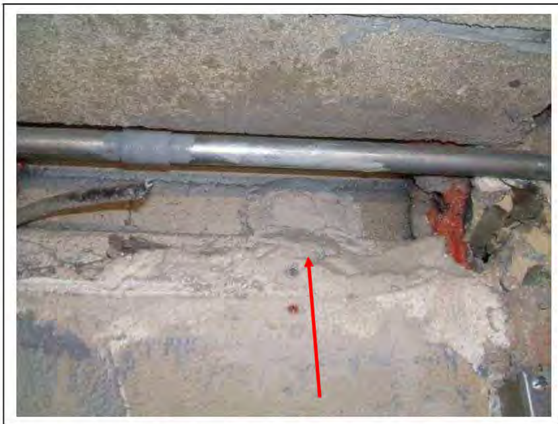
FIGURE 39: PRESUMED ASBESTOS BEHIND RENDER ON BRICK WALL IN PASSAGE , 2/238 - DESCRIPTION & RESULT OF ASSESSMENT (SAMPLE REF. P1&2(26))
