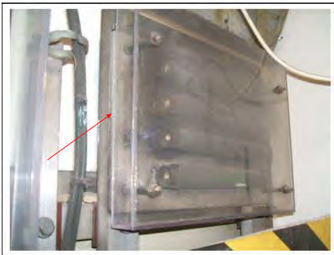
FIGURE 143: STRONGLY PRESUMED ASBESTOS IN CEMENT BOARD IN SWITCH ROOM E5, 3/662 - DESCRIPTION & RESULT OF ASSESSMENT (SAMPLE REF. SP1(2))
