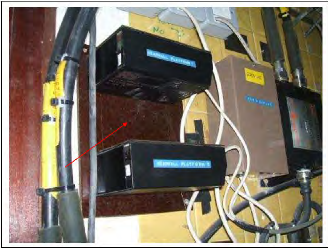
FIGURE 178: STRONGLY PRESUMED ASBESTOS IN SILUMINITE PANEL IN CER, 3/731 - DESCRIPTION & RESULT OF ASSESSMENT (SAMPLE REF. SP1(26))
