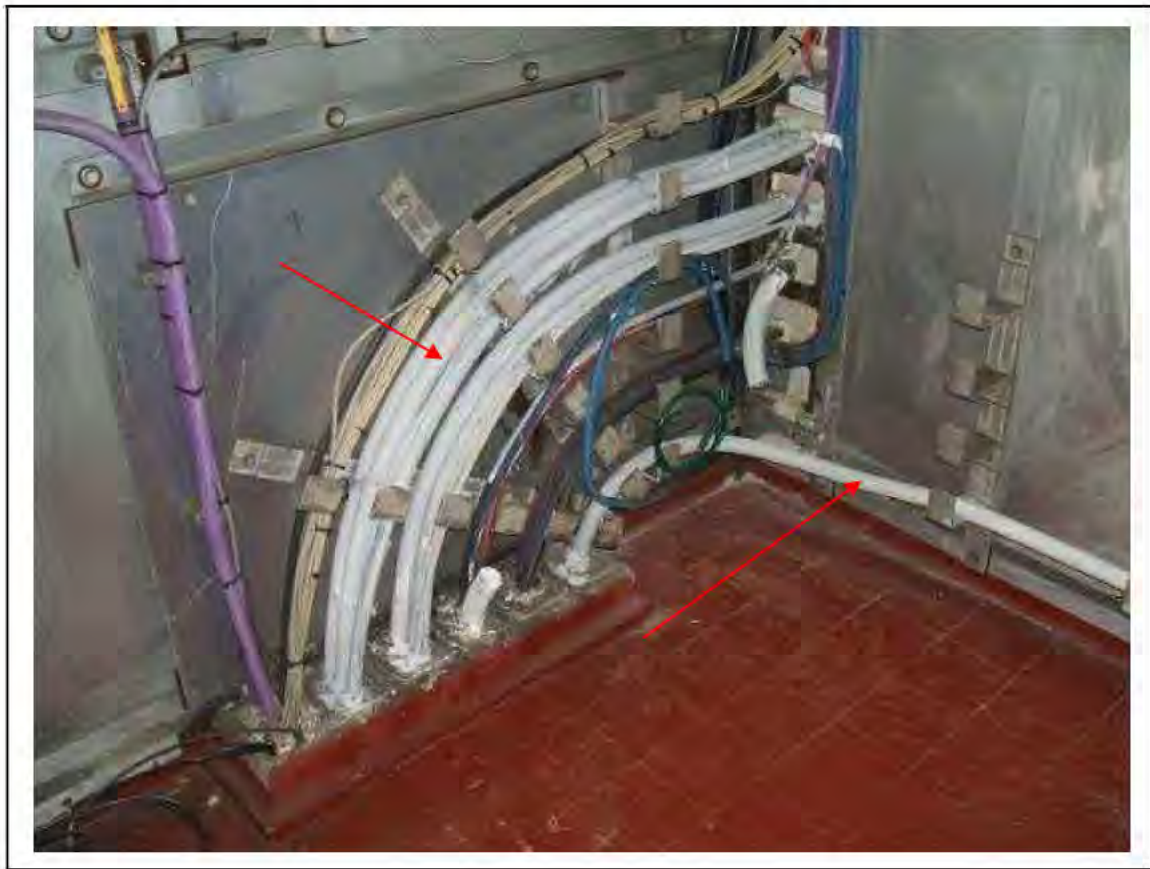
FIGURE 168: KNOWN ASBESTOS IN BRAIDED CABLES IN RELAY ROOM , 3/712 - DESCRIPTION & RESULT OF ASSESSMENT (SAMPLE REF. K1(43))
