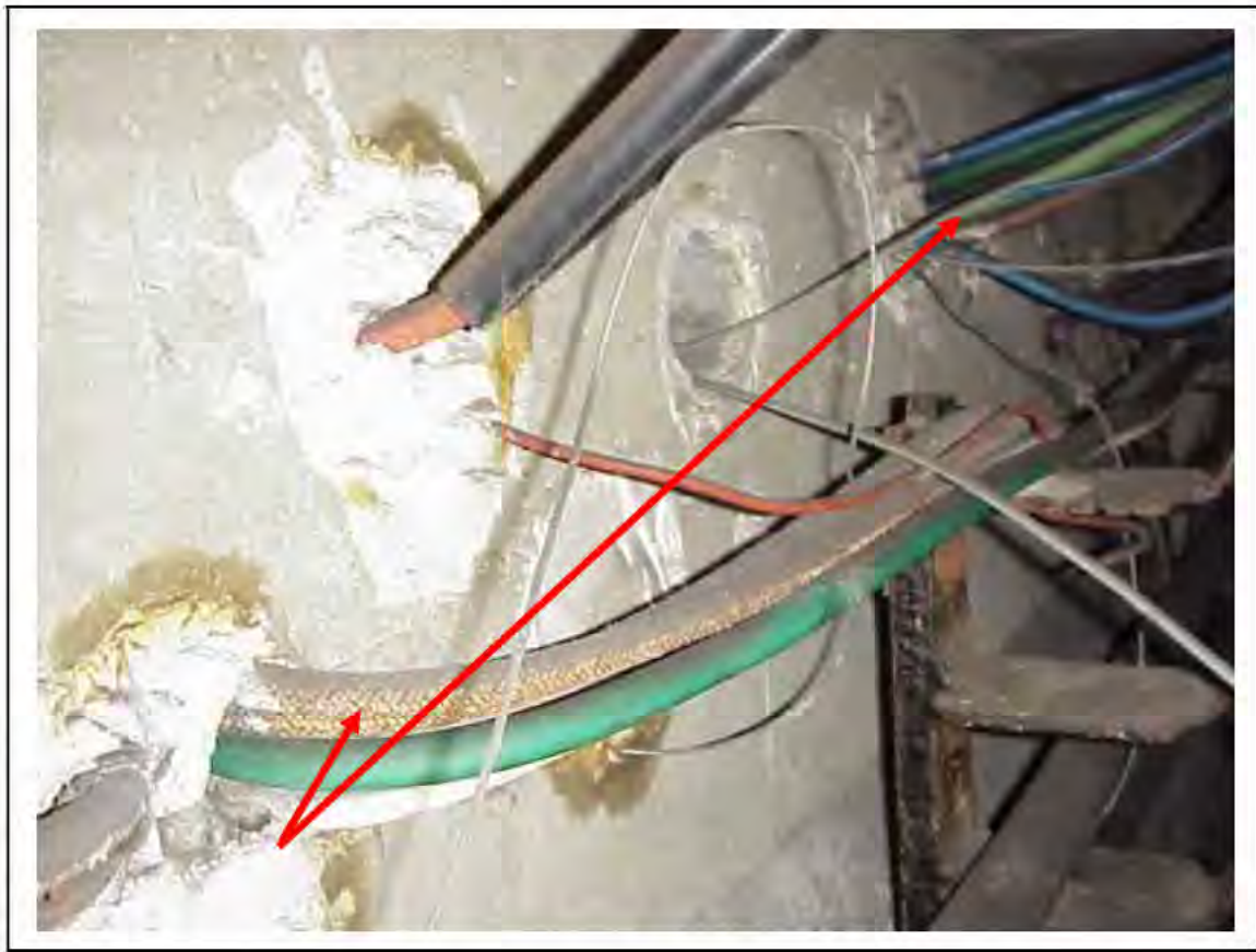
FIGURE 126: KNOWN ASBESTOS IN CABLES IN VICTORIA LINE, PLATFORM 2 INVERT, 3/262, 15M DOWN - DESCRIPTION & RESULT OF ASSESSMENT (SAMPLE REF. K1(32))
