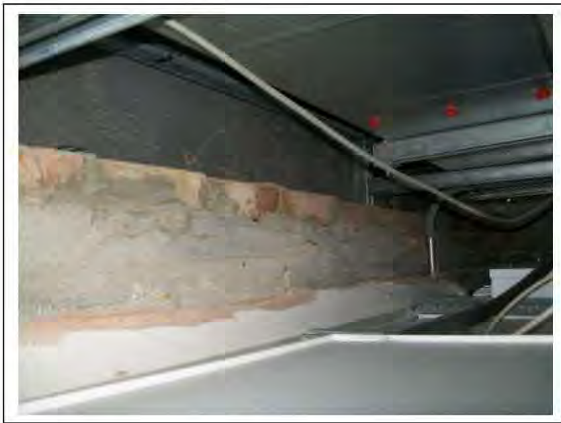
FIGURE 7: PRESUMED ASBESTOS IN RESIDUAL SPRAY INSULATION WITHIN WALL CAVITY IN OFFICE , 2/031 - DESCRIPTION & RESULT OF ASSESSMENT (SAMPLE REF. P1&2(7))
