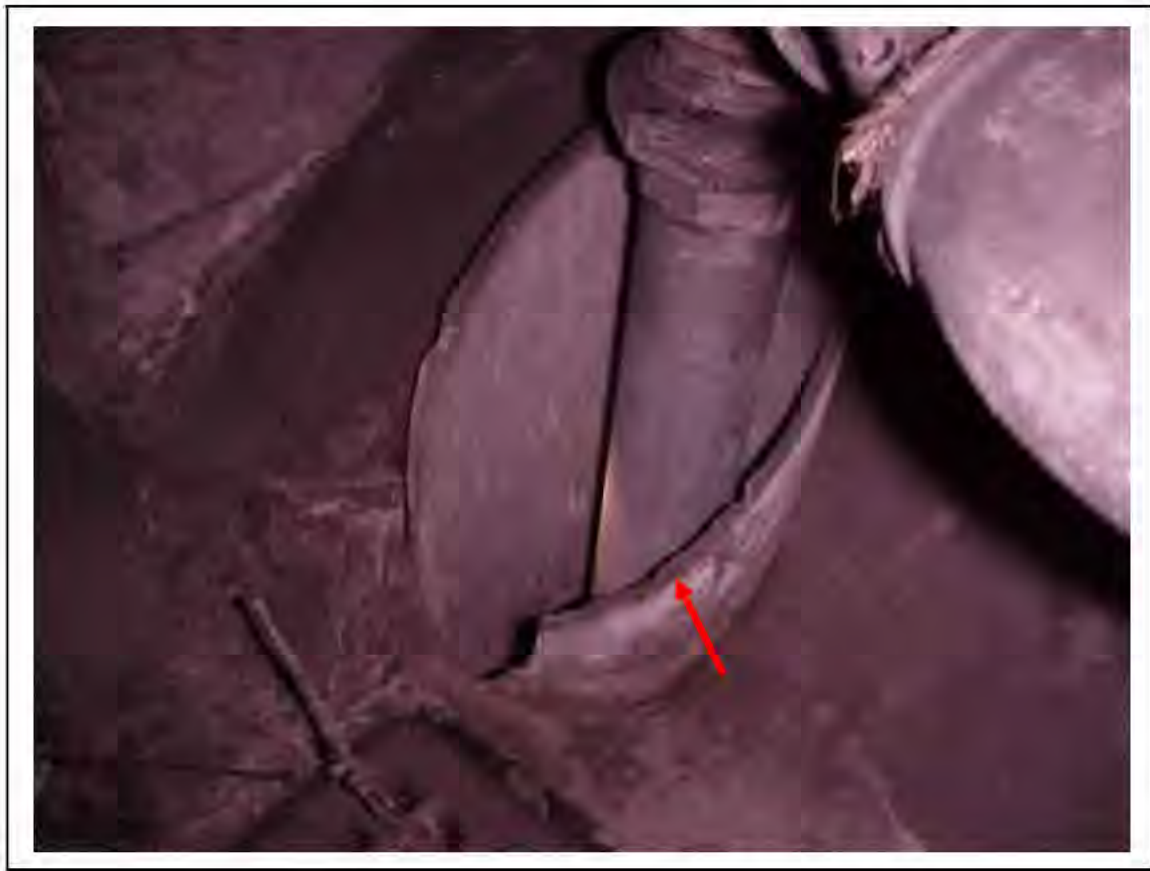
FIGURE 115: CONFIRMED ASBESTOS IN CABLE SLEEVES IN VICTORIA LINE, PLATFORM 1 INVERT, 3/261, 10M ON HALF WAY - DESCRIPTION & RESULT OF ASSESSMENT (SAMPLE REF. 034219/10)
