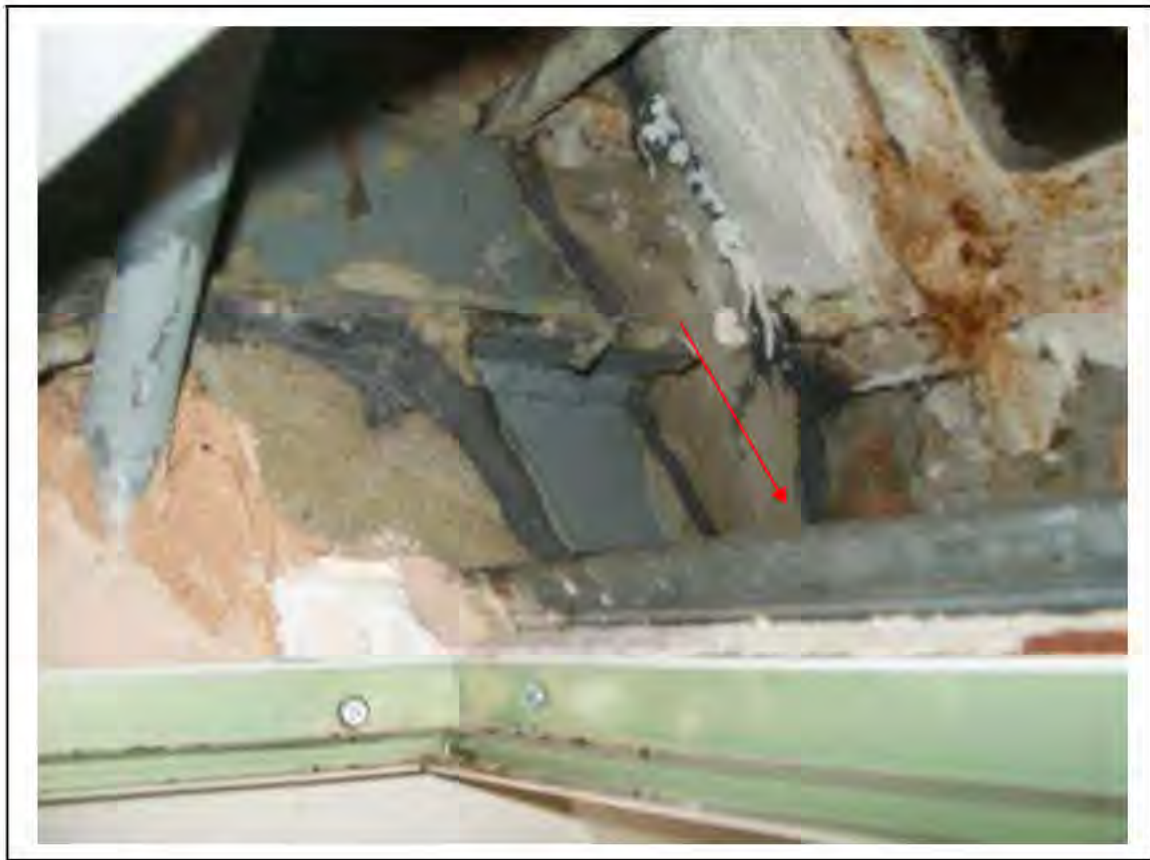
FIGURE 75: KNOWN ASBESTOS IN CELLACTITE CORRUGATED SHEETING IN MESS ROOM , 3/053 - DESCRIPTION & RESULT OF ASSESSMENT (SAMPLE REF. K1(9))
