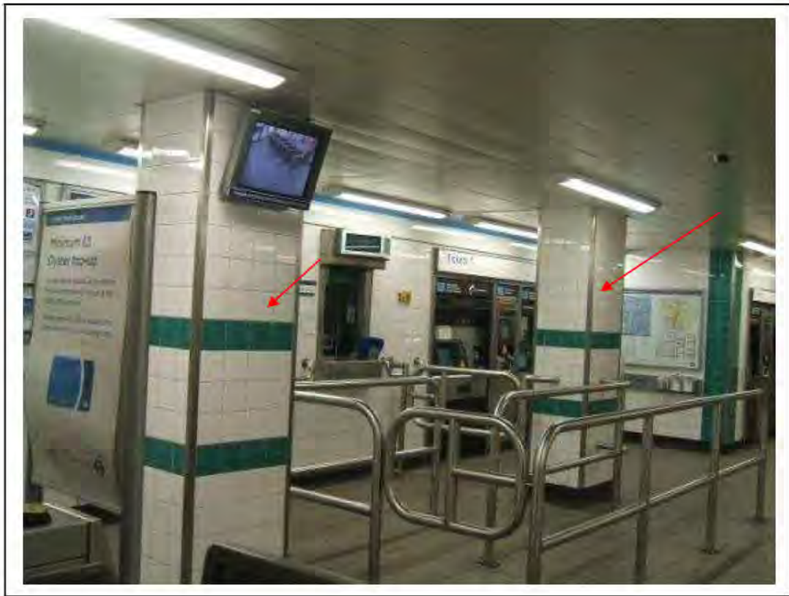
FIGURE 1: PRESUMED ASBESTOS IN RESIDUE IN PILLARS IN TICKET HALL , 2/001 - DESCRIPTION & RESULT OF ASSESSMENT (SAMPLE REF. P1&2(1))
