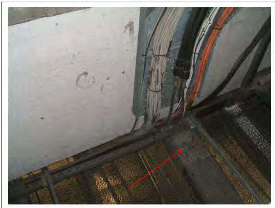
FIGURE 194: PRESUMED ASBESTOS IN RESIDUES TO LIGHTING BOXES IN VENT SHAFT , 3/902 - DESCRIPTION & RESULT OF ASSESSMENT (SAMPLE REF. P1&2(59))
