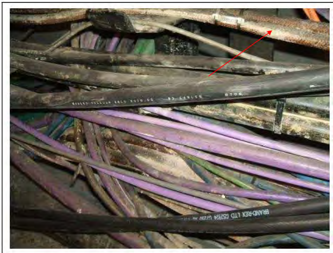
FIGURE 184: STRONGLY PRESUMED ASBESTOS IN BRAIDED CABLES IN CABLE SHAFT , 3/786 - DESCRIPTION & RESULT OF ASSESSMENT (SAMPLE REF. SP1(28))
