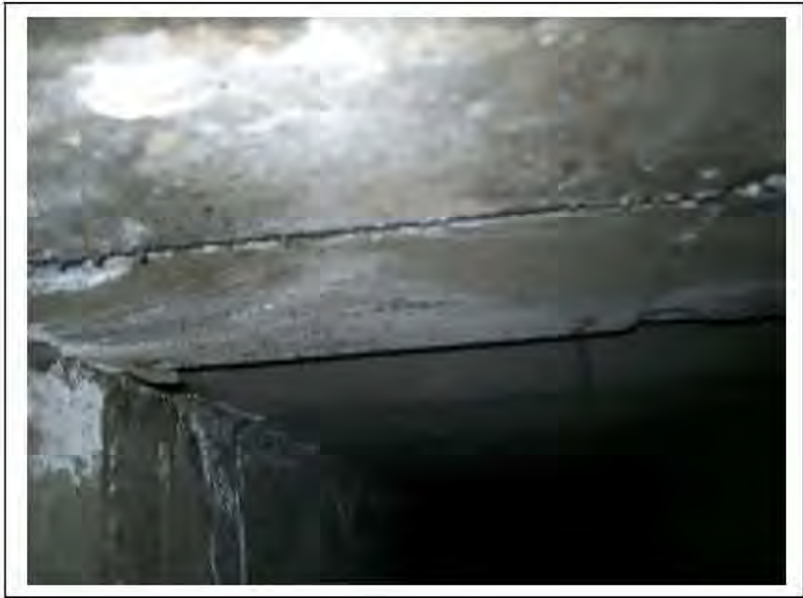
FIGURE 83: CONFIRMED ASBESTOS IN DUCTS BY ESCALATORS IN LMC, 3/161 - DESCRIPTION & RESULT OF ASSESSMENT (SAMPLE REF. 120445/180812/02)
