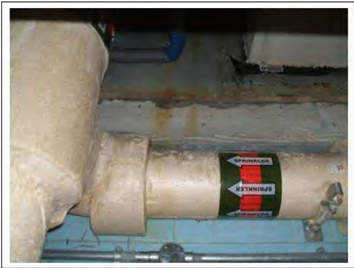
FIGURE 63: PRESUMED ASBESTOS IN RESIDUES WITHIN EXTERNAL WALL IN SERVICE VOID , 2/901 - DESCRIPTION & RESULT OF ASSESSMENT (SAMPLE REF. P1&2(47))
