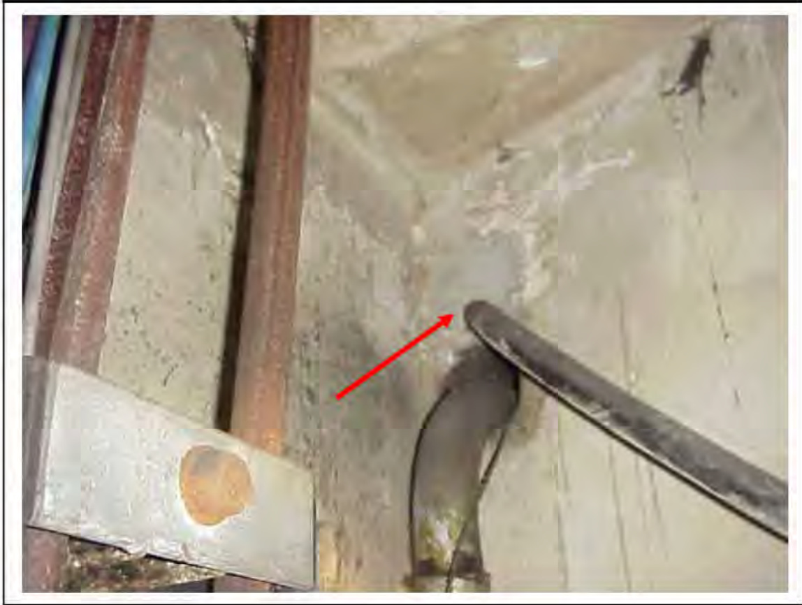
FIGURE 120: CONFIRMED ASBESTOS IN CABLE SLEEVES IN VICTORIA LINE, PLATFORM 2 INVERT, 3/262, DOWN HATCH NEAR 3/712 - DESCRIPTION & RESULT OF ASSESSMENT (SAMPLE REF. 034219/1)
