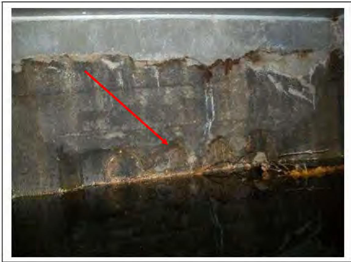
FIGURE 99: CONFIRMED ASBESTOS IN CEMENT DUCT IN CROSS PASSAGE FLOOR DUCT, 3/208 - DESCRIPTION & RESULT OF ASSESSMENT (SAMPLE REF. 120445/200812/01)
