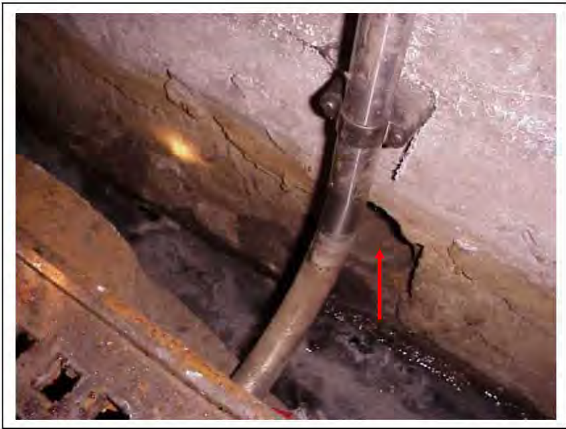
FIGURE 128: CONFIRMED ASBESTOS IN CABLE SLEEVES IN VICTORIA LINE, PLATFORM 2 INVERT, 3/262, 10M ON HALFWAY - DESCRIPTION & RESULT OF ASSESSMENT (SAMPLE REF. SAME AS 034219/5)
