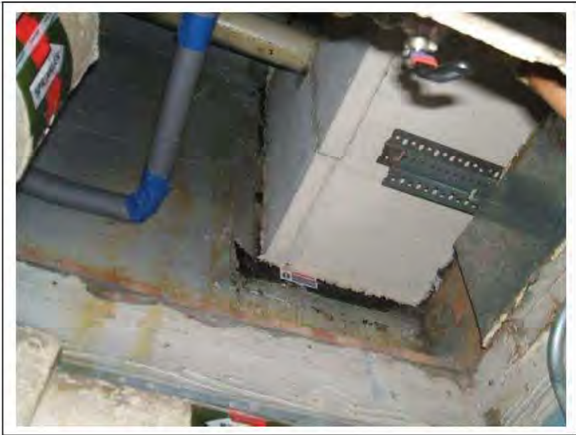
FIGURE 62: PRESUMED ASBESTOS IN RESIDUES WHERE BEAM ENTERS EXTERNAL WALL IN SERVICE VOID , 2/901 - DESCRIPTION & RESULT OF ASSESSMENT (SAMPLE REF. P1&2(46))
