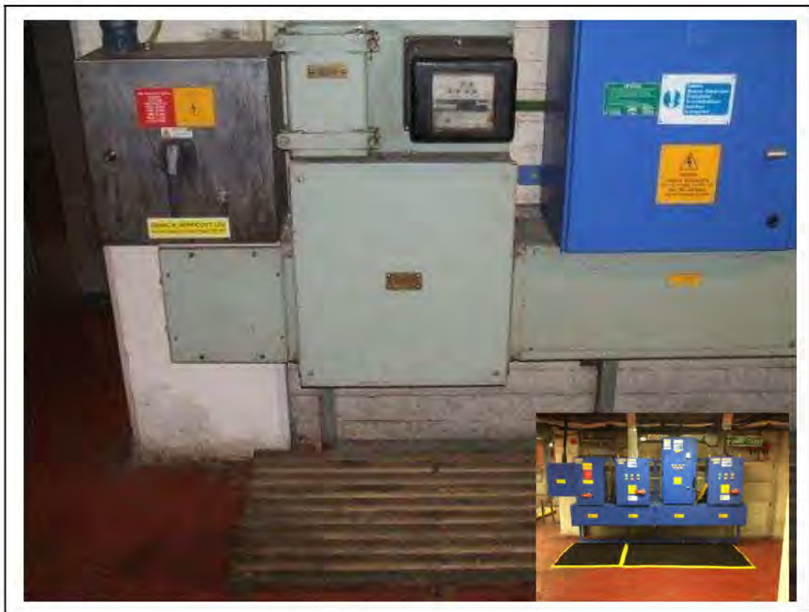
FIGURE 21: PRESUMED ASBESTOS IN WATT HOUR METER / FUSEBOARD IN UMC, 2/151 - DESCRIPTION & RESULT OF ASSESSMENT (SAMPLE REF. P1(1))
