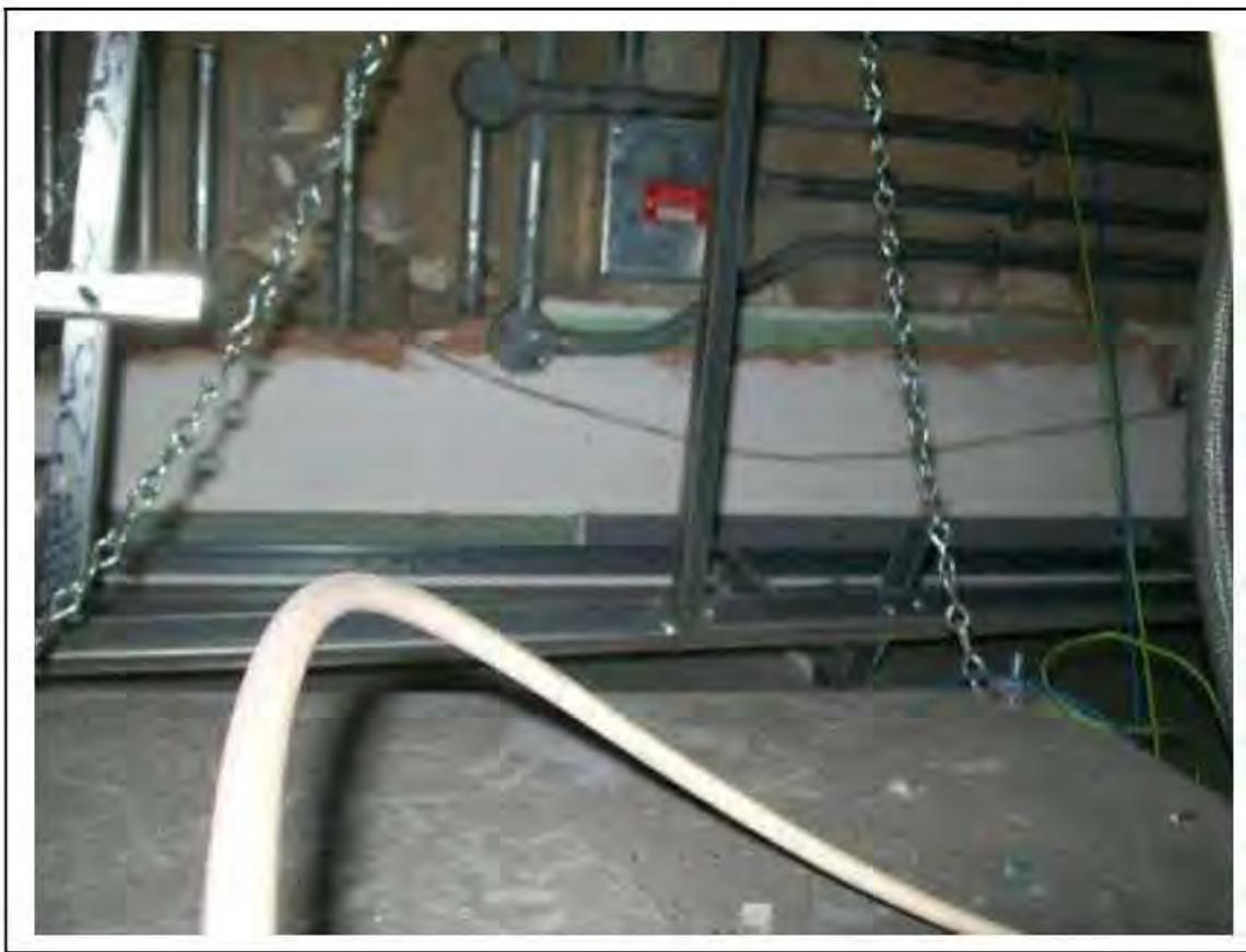
FIGURE 61: PRESUMED ASBESTOS IN RESIDUES WITHIN WALL CAVITY IN OFFICE , 2/801 - DESCRIPTION & RESULT OF ASSESSMENT (SAMPLE REF. P1&2(45))
