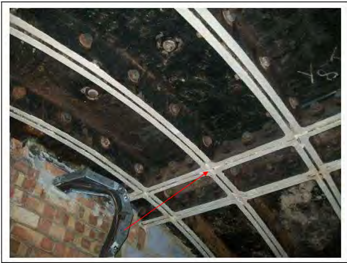
FIGURE 95: CONFIRMED ASBESTOS IN CAULKING IN PASSAGE , 3/207 - DESCRIPTION & RESULT OF ASSESSMENT (SAMPLE REF. AS 120445/150812/03)
