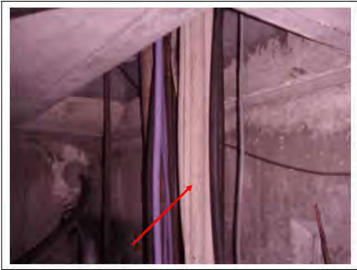
FIGURE 109: KNOWN ASBESTOS IN CABLES IN VICTORIA LINE, PLATFORM 1 INVERT, 3/261, DOWN HATCH NEAR 3/711 - DESCRIPTION & RESULT OF ASSESSMENT (SAMPLE REF. K1(25))
