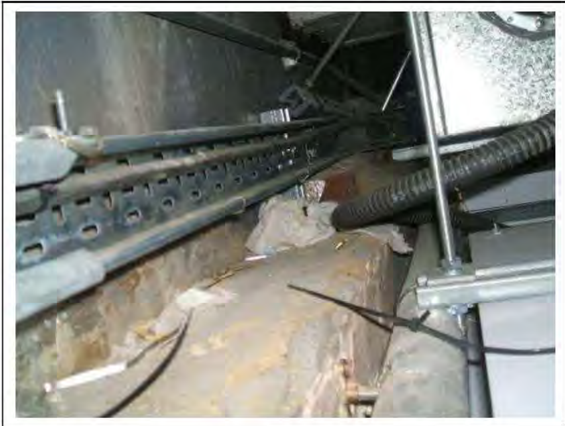
FIGURE 4: PRESUMED ASBESTOS IN EXTERNAL CAVITY WALL LIKELY RESIDUES IN CAVITY BEHIND TICKET OFFICE CORRIDOR, 2/011 - DESCRIPTION & RESULT OF ASSESSMENT (SAMPLE REF. P1&2(4))
