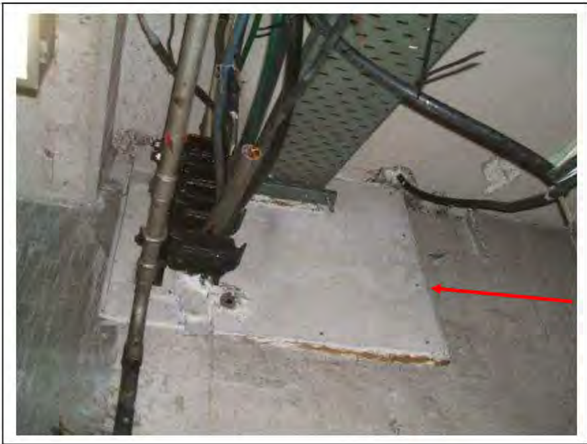
FIGURE 27: PRESUMED ASBESTOS BEHIND SUPALUX PANEL IN UMC, 2/151 - DESCRIPTION & RESULT OF ASSESSMENT (SAMPLE REF. P1(5))
