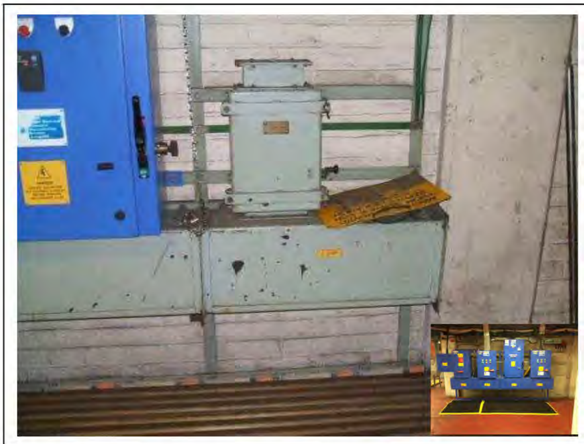
FIGURE 23: PRESUMED ASBESTOS IN AUXILIARY PLANT BOX IN UMC, 2/151 - DESCRIPTION & RESULT OF ASSESSMENT (SAMPLE REF. P1(3))
