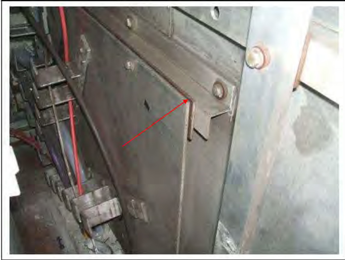
FIGURE 161: STRONGLY PRESUMED ASBESTOS IN SILUMINITE PACKING STRIPS IN IMR (CORRIDOR TO PLATFORM 2), 3/706 - DESCRIPTION & RESULT OF ASSESSMENT (SAMPLE REF. SP1(13))
