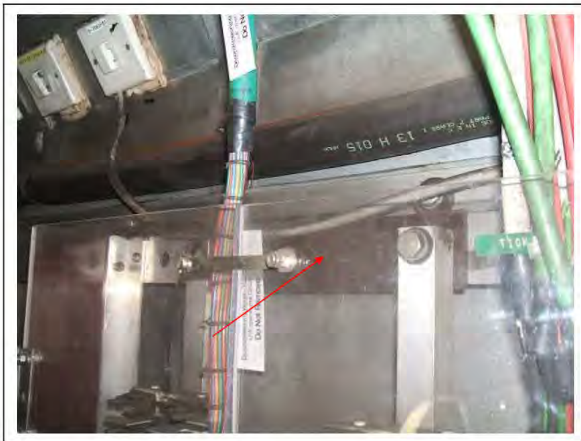
FIGURE 158: STRONGLY PRESUMED ASBESTOS IN SILUMINITE LABELS IN IMR (CORRIDOR TO PLATFORM 2), 3/706 - DESCRIPTION & RESULT OF ASSESSMENT (SAMPLE REF. SP1(11))
