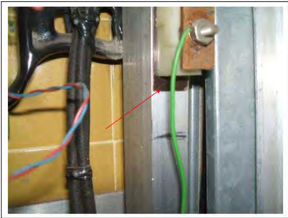
FIGURE 180: STRONGLY PRESUMED ASBESTOS IN SILUMINITE STRIP IN CER , 3/731 - DESCRIPTION & RESULT OF ASSESSMENT (SAMPLE REF. SP1(27))
