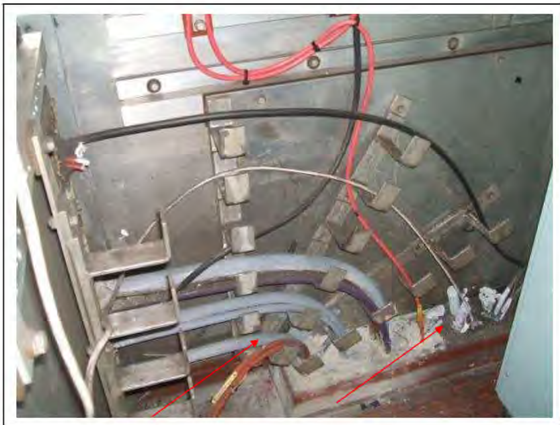
FIGURE 156: KNOWN ASBESTOS IN BRAIDED CABLES IN IMR (CORRIDOR TO PLATFORM 2), 3/706 - DESCRIPTION & RESULT OF ASSESSMENT (SAMPLE REF. K1(39))
