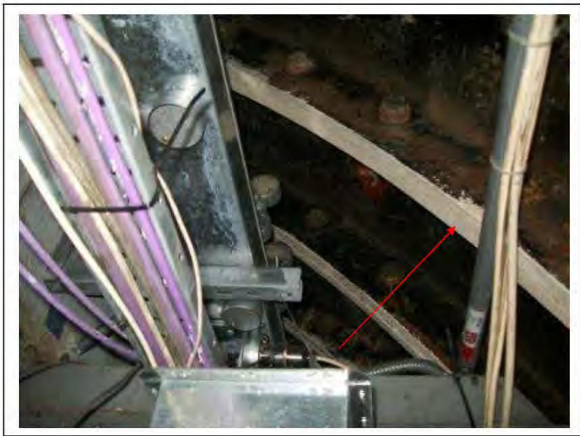
FIGURE 101: CONFIRMED ASBESTOS IN CAULKING IN CORRIDOR , 3/236 - DESCRIPTION & RESULT OF ASSESSMENT (SAMPLE REF. SAME AS 120445/150812/03)
