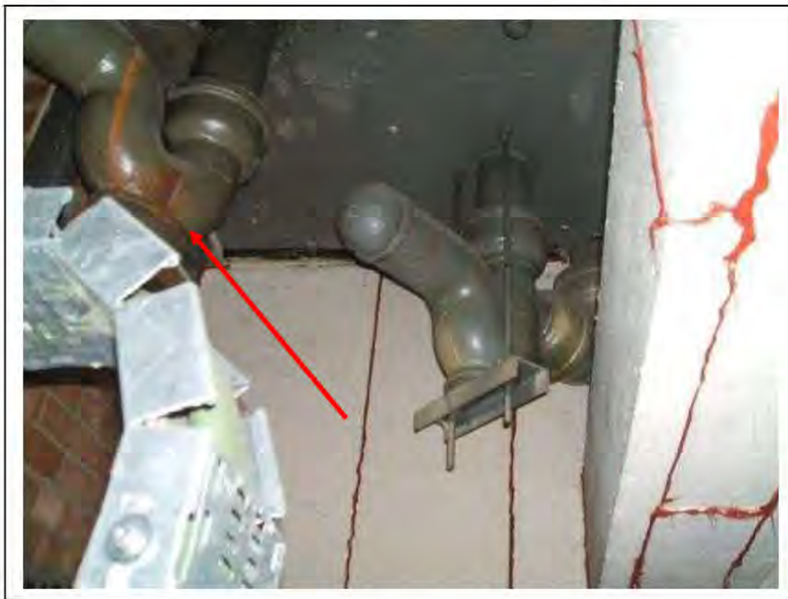
FIGURE 15: PRESUMED ASBESTOS IN RESIDUE AROUND SOIL PIPE IN UMC ACCESS , 2/151 - DESCRIPTION & RESULT OF ASSESSMENT (SAMPLE REF. P1&2(14))
