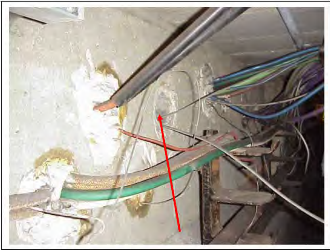
FIGURE 125: CONFIRMED ASBESTOS IN CABLE SLEEVES IN VICTORIA LINE, PLATFORM 2 INVERT, 3/262, 15M DOWN - DESCRIPTION & RESULT OF ASSESSMENT (SAMPLE REF. 034219/4)
