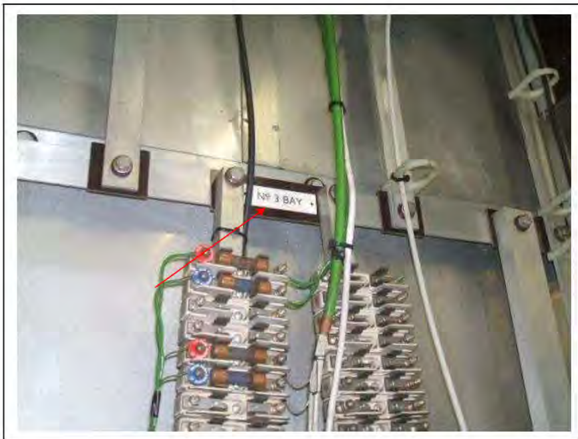
FIGURE 173: STRONGLY PRESUMED ASBESTOS IN SILUMINITE IN RELAY ROOM , 3/712 - DESCRIPTION & RESULT OF ASSESSMENT (SAMPLE REF. SP1(22))
