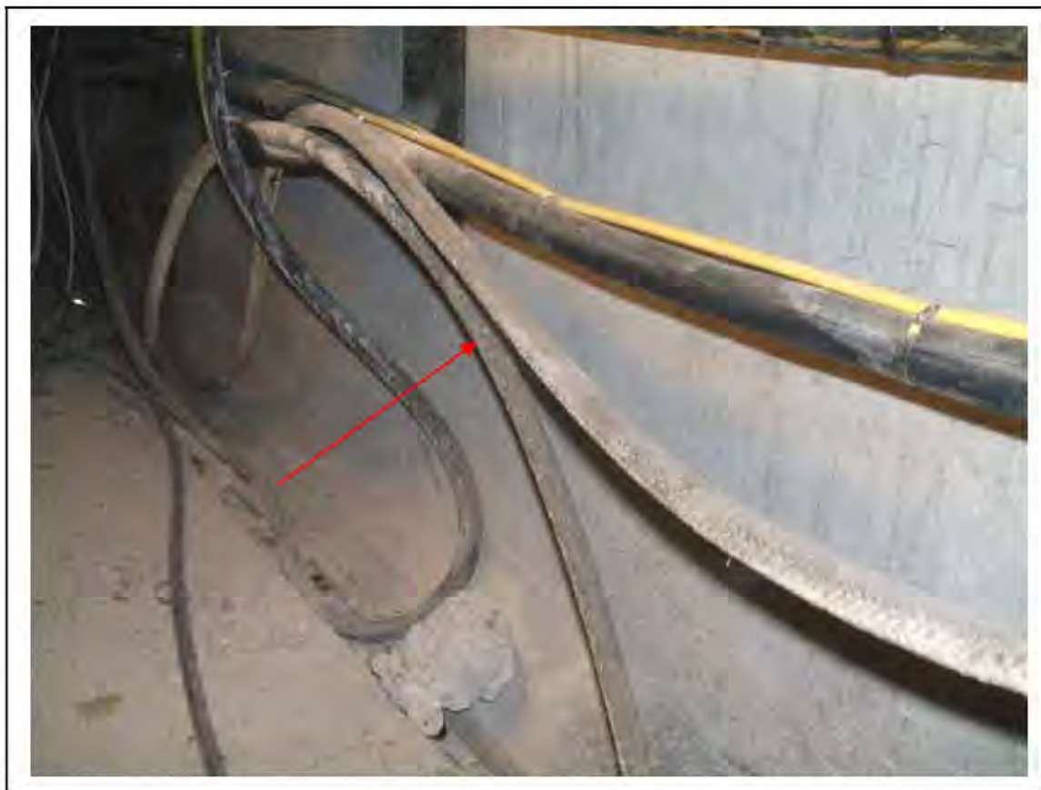
FIGURE 189: KNOWN ASBESTOS IN BRAIDED CABLES IN CABLE SHAFT , 3/787 - DESCRIPTION & RESULT OF ASSESSMENT (SAMPLE REF. K1(49))
