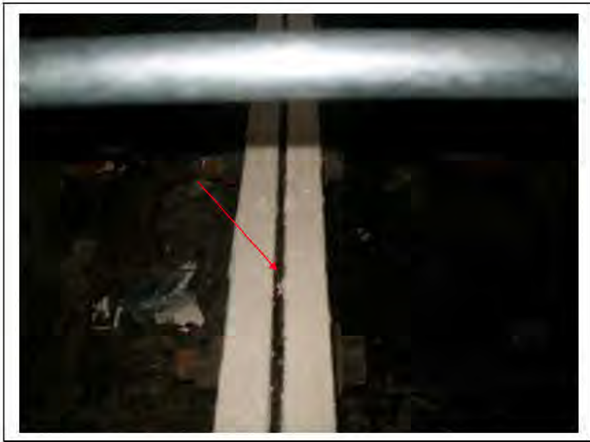
FIGURE 74: CONFIRMED ASBESTOS IN CAULKING IN MESS ROOM , 3/053 - DESCRIPTION & RESULT OF ASSESSMENT (SAMPLE REF. 120445/150812/03)
